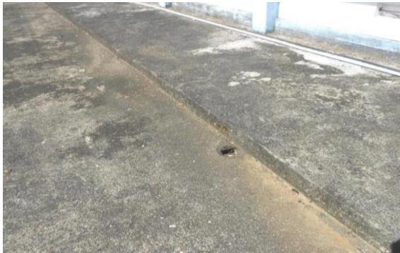
Chocked Rain water drain
