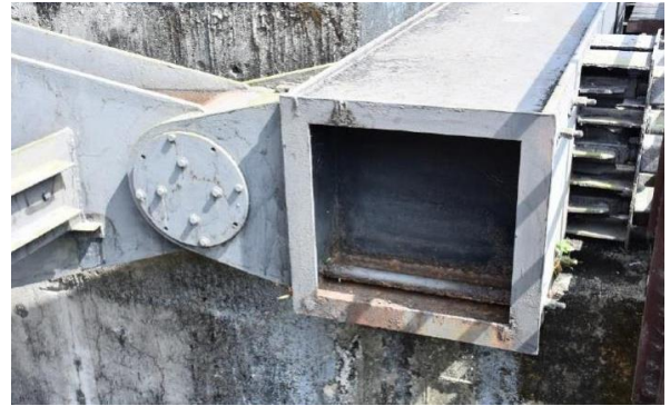
Radial gate-Yoke Girder- water deposit & rusting of Trunnion bolt
