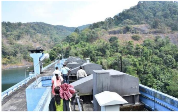
Requirement of roof top at hoist operating area
