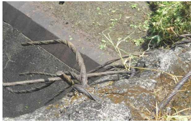
Damaged right side training wall
