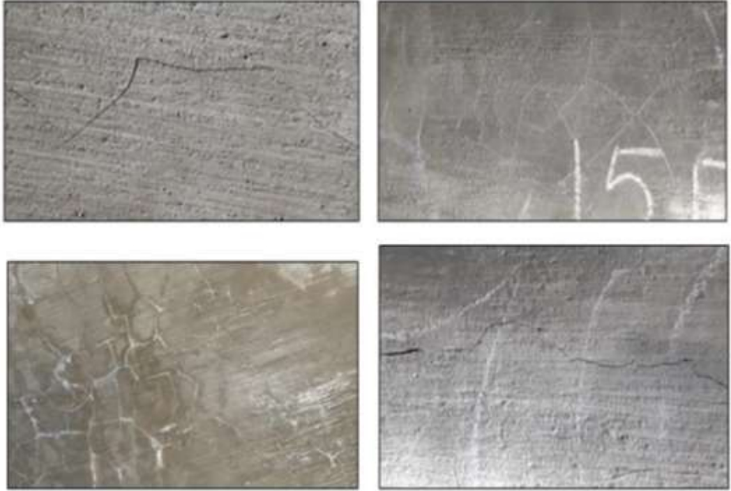
Cracks in the Gallery of Cheruthoni
