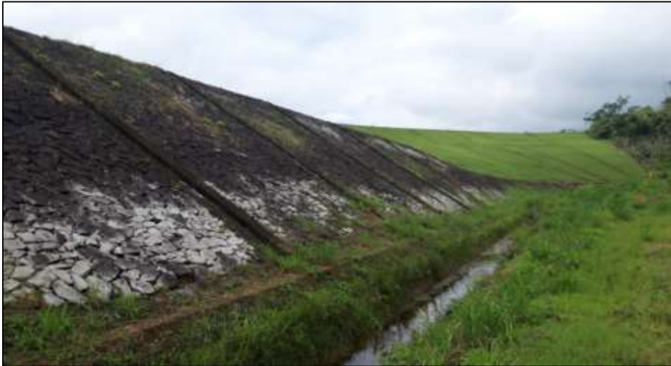
KA dam – Rectification is required for damaged surface drains
