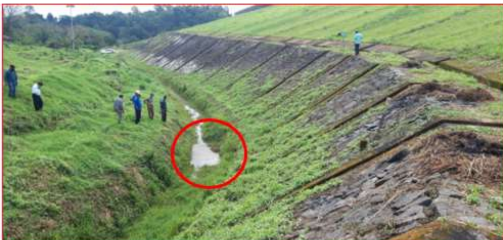
Boiling observed at toe of KA dam
