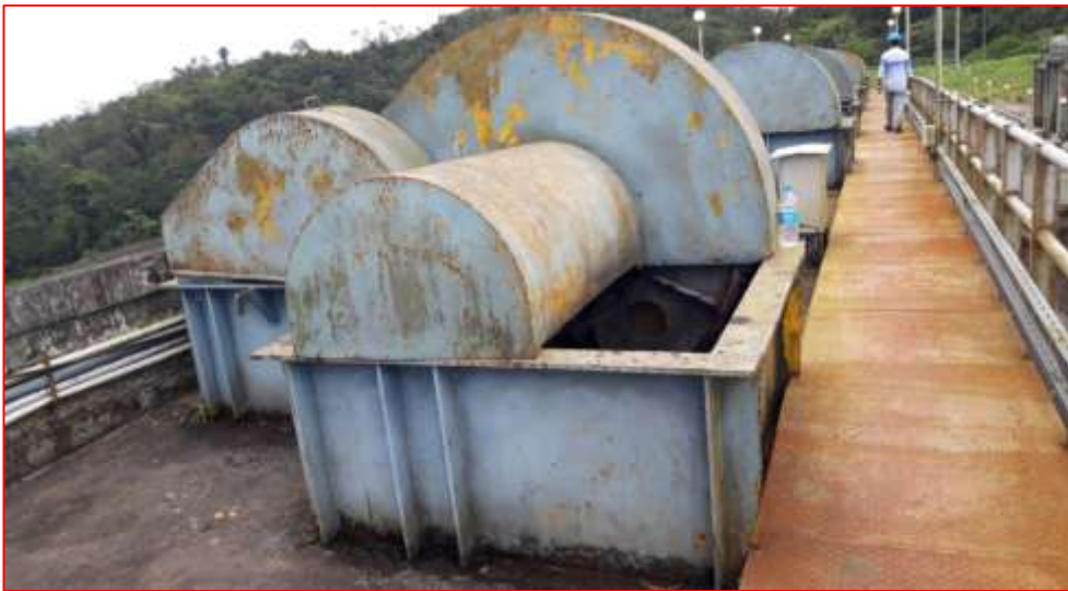
Hoist protection corroded – Needs roofing
