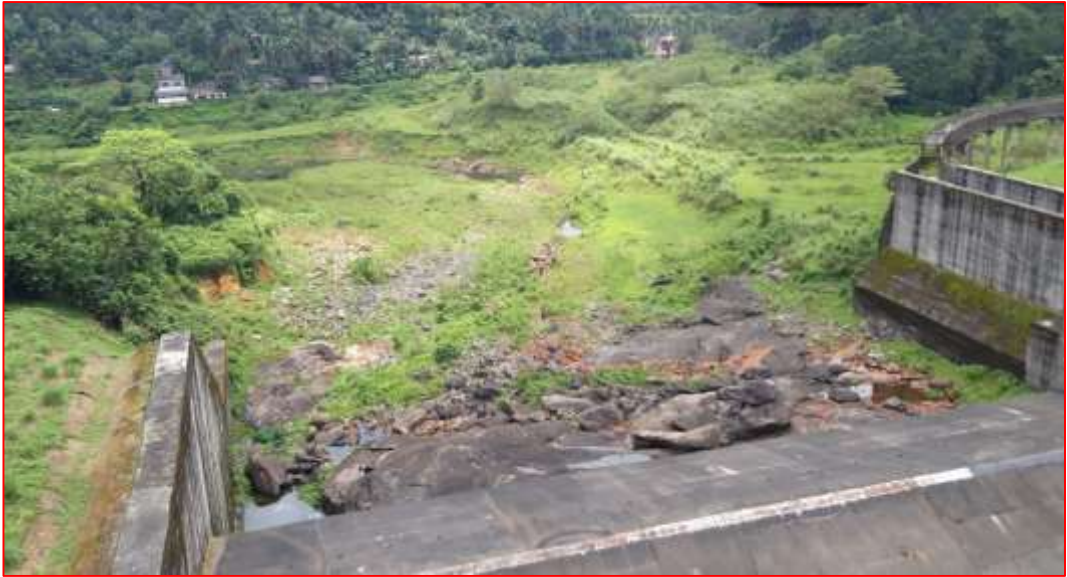
Slope protection d/s of spillway eroded – Protective works to be extended
