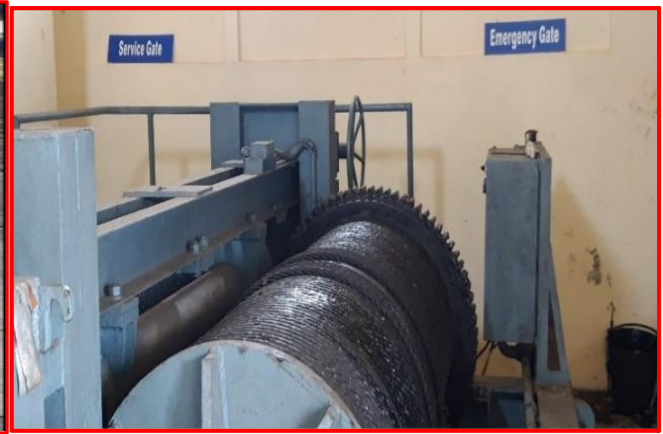
Hoist of Emergency/Service Gate- needs overhauling
