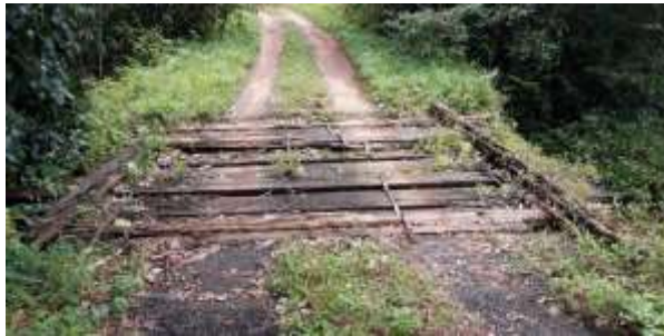
Damaged wooden bridge on the way to IC tunnel control shaft
