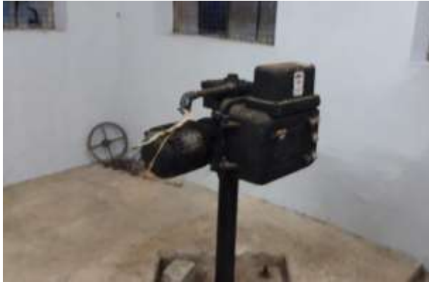
Motor for operating hollow jet valve – Pamba Dam – faulty electrical connections
