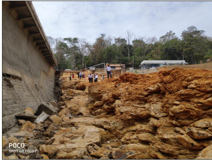
Eroded foundation portion at downstream face
