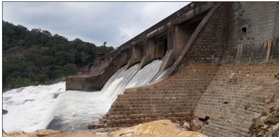
Damaged training wall
