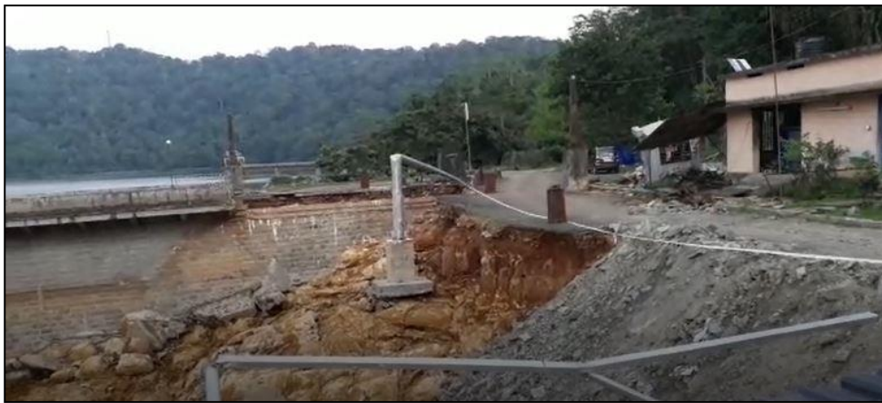
Damaged portion of Access road to dam top
