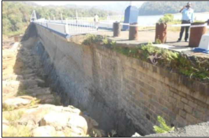
Eroded portion of d/s side abutment at left bank of dam
