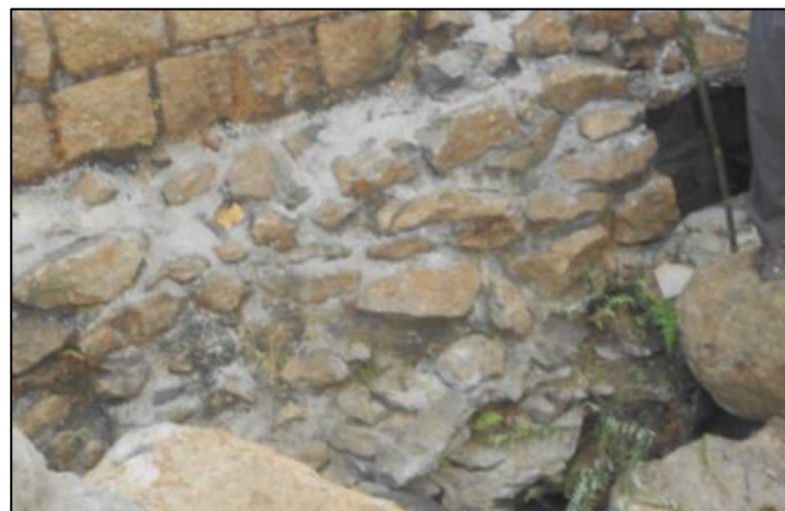
Damaged foundation at downstream
