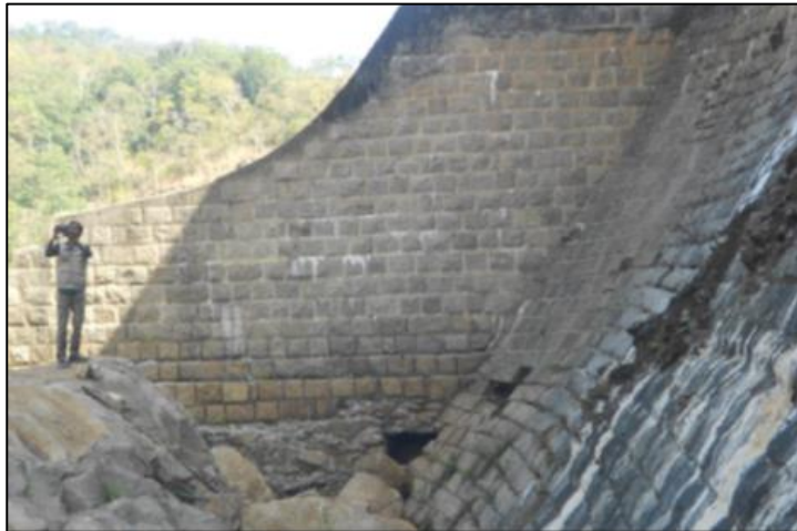
Damaged portion of the abutment at d/s side of dam
