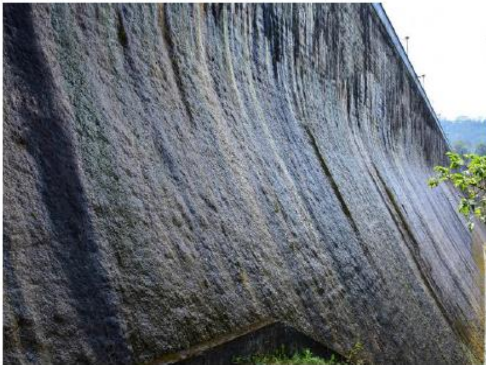
Wetting at the downstream of dam body
