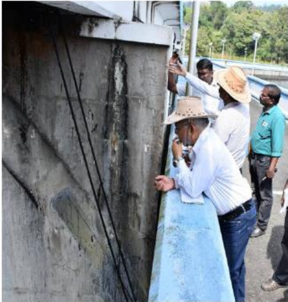
Crack near Spillway Gate pier – Inspection by DSRP
