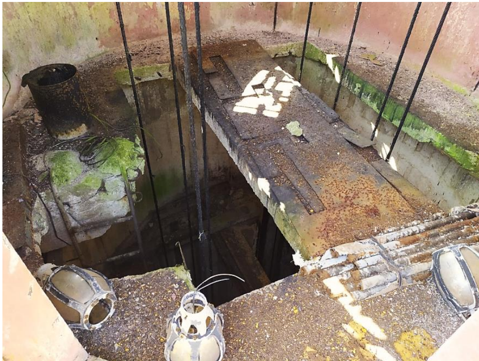
Fig 2.11 Anayirankal dam Emergency & Service gates hoist
