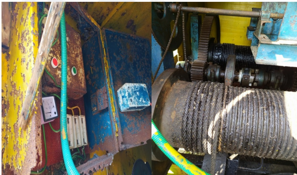
Fig 2.12 Emergency & Service gates hoist mechanism
