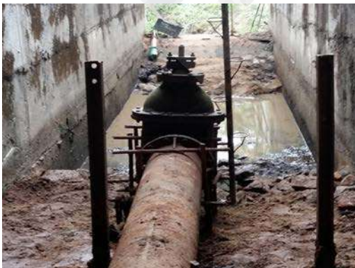
Fig 2.4a River Outlet Valve
