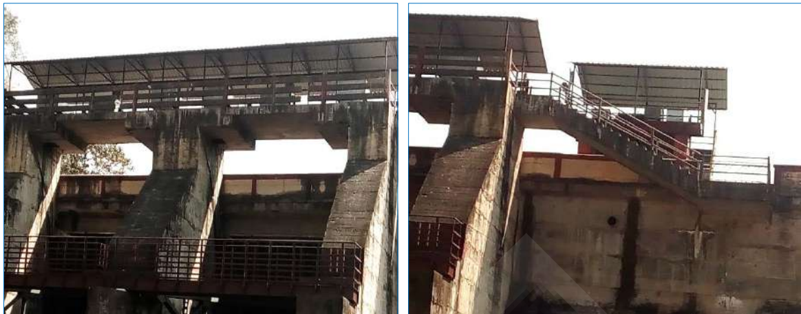
Erattayar dam - Hoist bridge for Spillway Radial gates and Emergency gate of river outlet – Roofing
