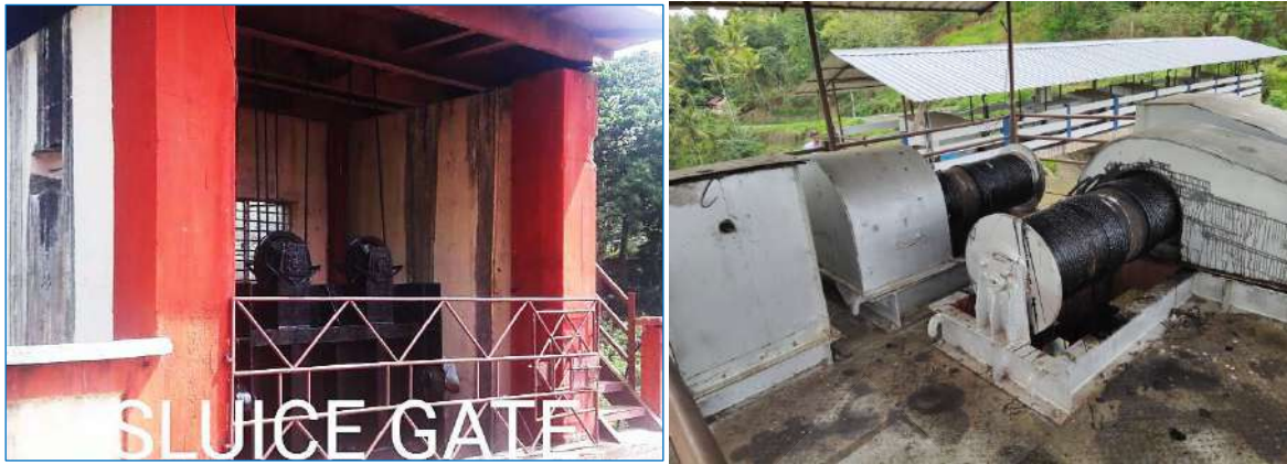
Fig 2.5b Sluice Gate and Hoist Motor
