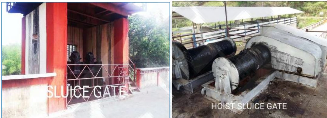
Erattayar dam River outlet Gate and Hoist
