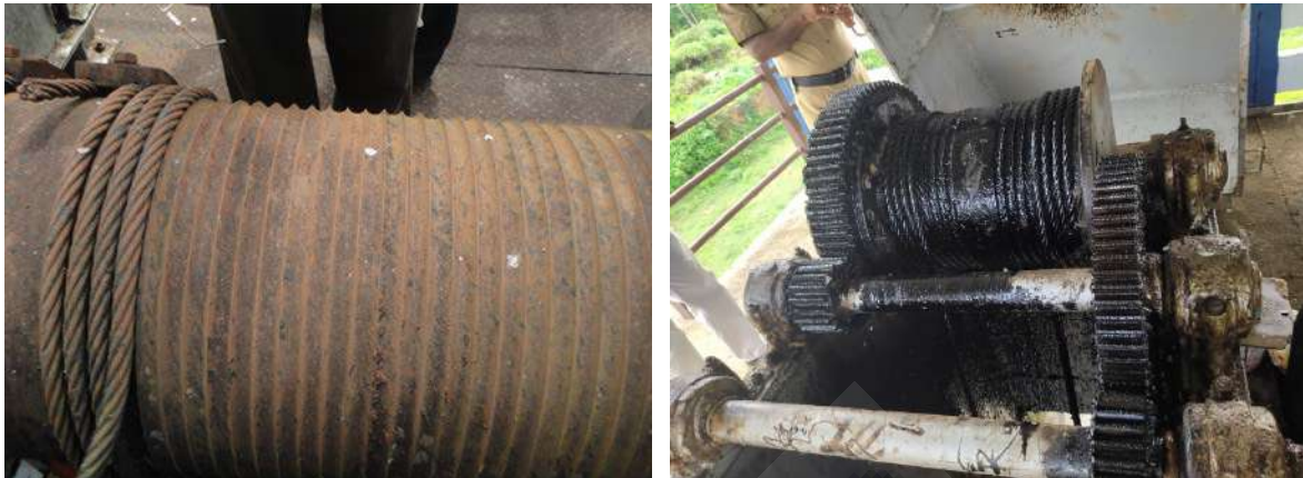
Erattayar dam Radial Gate hoist mechanism
