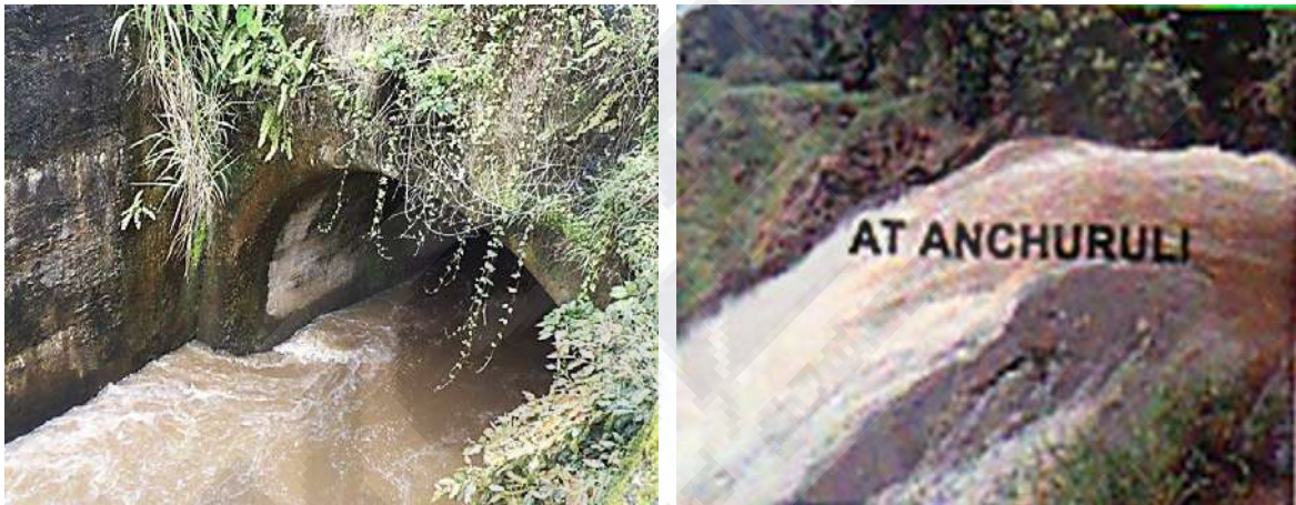
Fig 2.12 Erattayar Dam Diversion Tunnel to Idukki reservoir (Entry from Leading Channel and Exit at Anchuruli)
