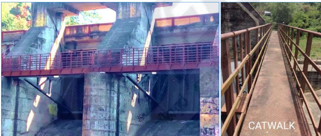
Erattayar dam catwalk d/s of spillway for maintenance of radial gate trunnion
