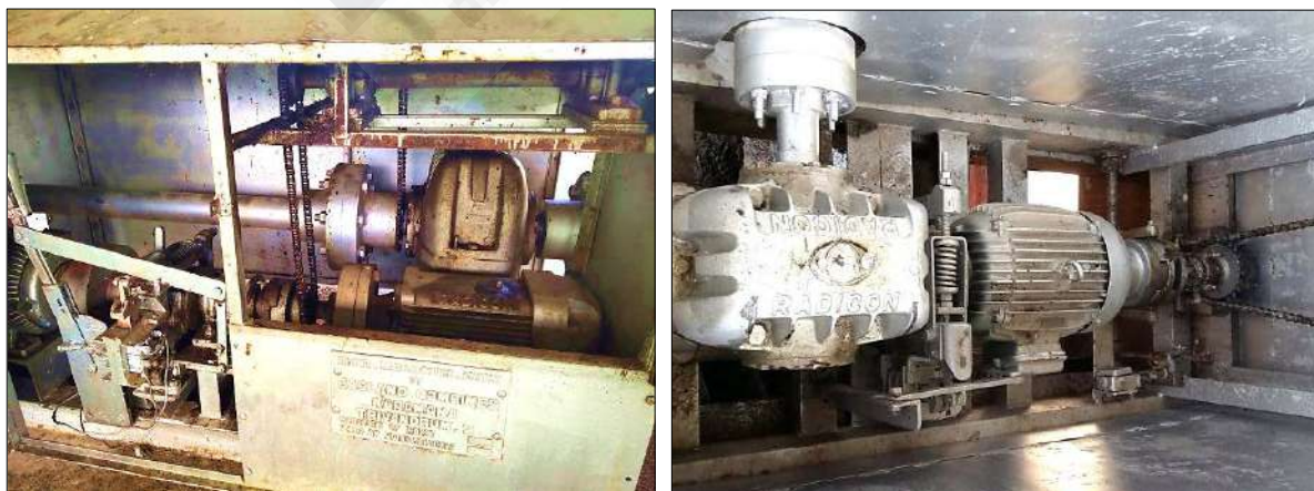
Fig 2.9b Radial Gates hoist motor
