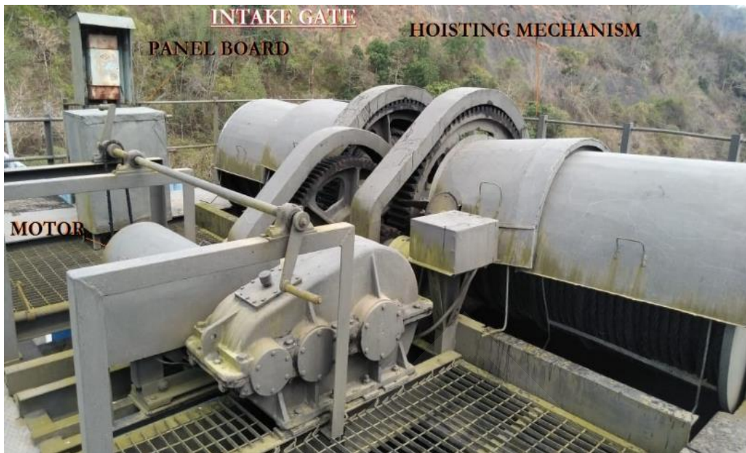
Fig 2.11 Idamalayar Dam Intake Gate Hoist Mechanism
