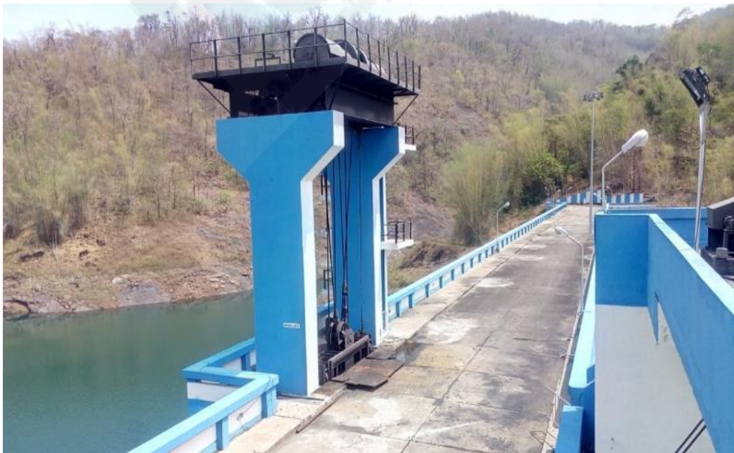
Fig 2.10 Idamalayar Dam Vertical Gate
