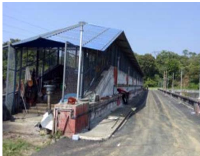
Supply and Erection of Roofing to hoist of Anathodu Dam radial gate
