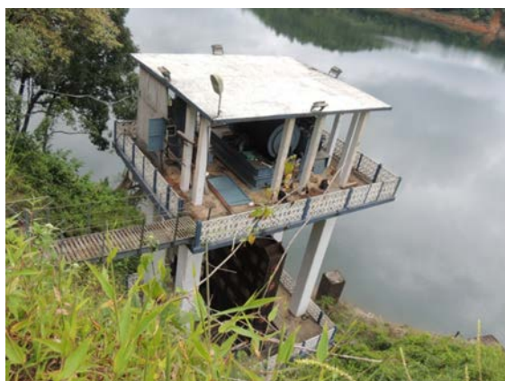
PROTECTIVE ROOFING TO INTAKE BUILDING (BEFORE)
