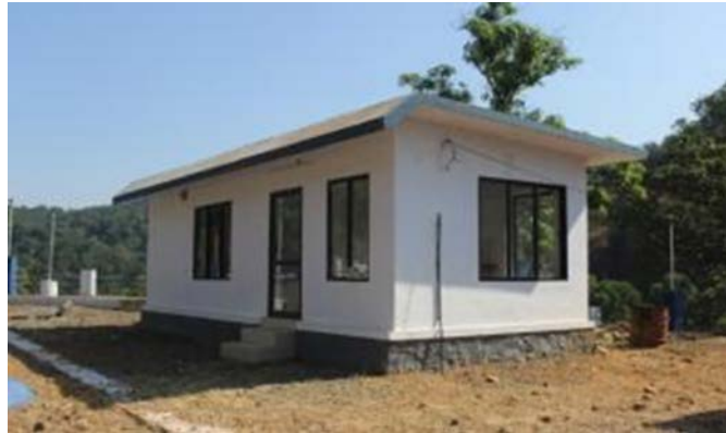
Monitoring cabin – Final stage
