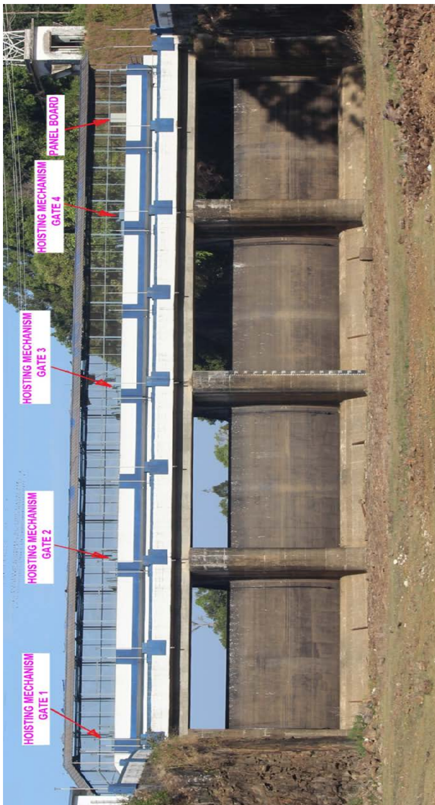
Fig 2.4 Hoisting Mechanism and Control Panel for Anathodu Dam
