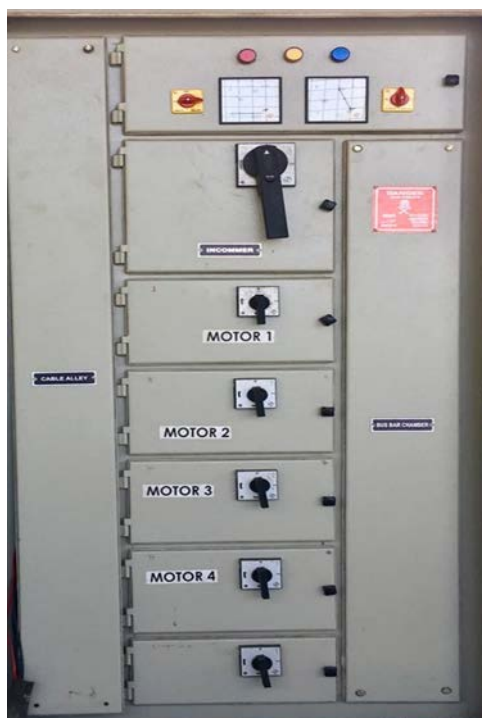
Fig 2.5 Control panel of the radial gates
