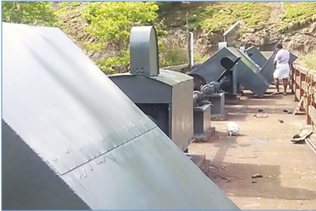
Fig 2.8 Radial Gates hoist mechanism
