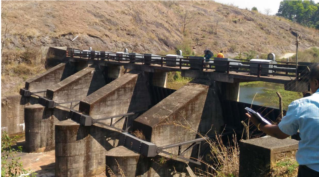
Fig 2.6 View of Radial Gates hoisting Mechanism from downstream
