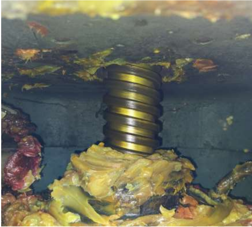
Fig 2.8 Spillway gate hoisting gear
