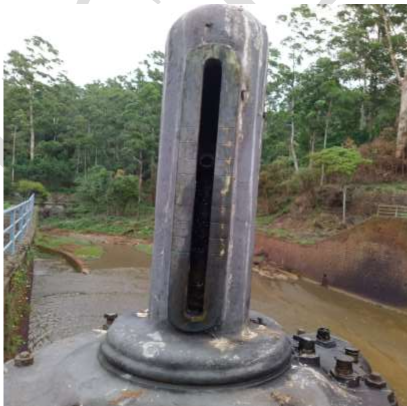
Fig 2.13 Disperser valve hoist dial
