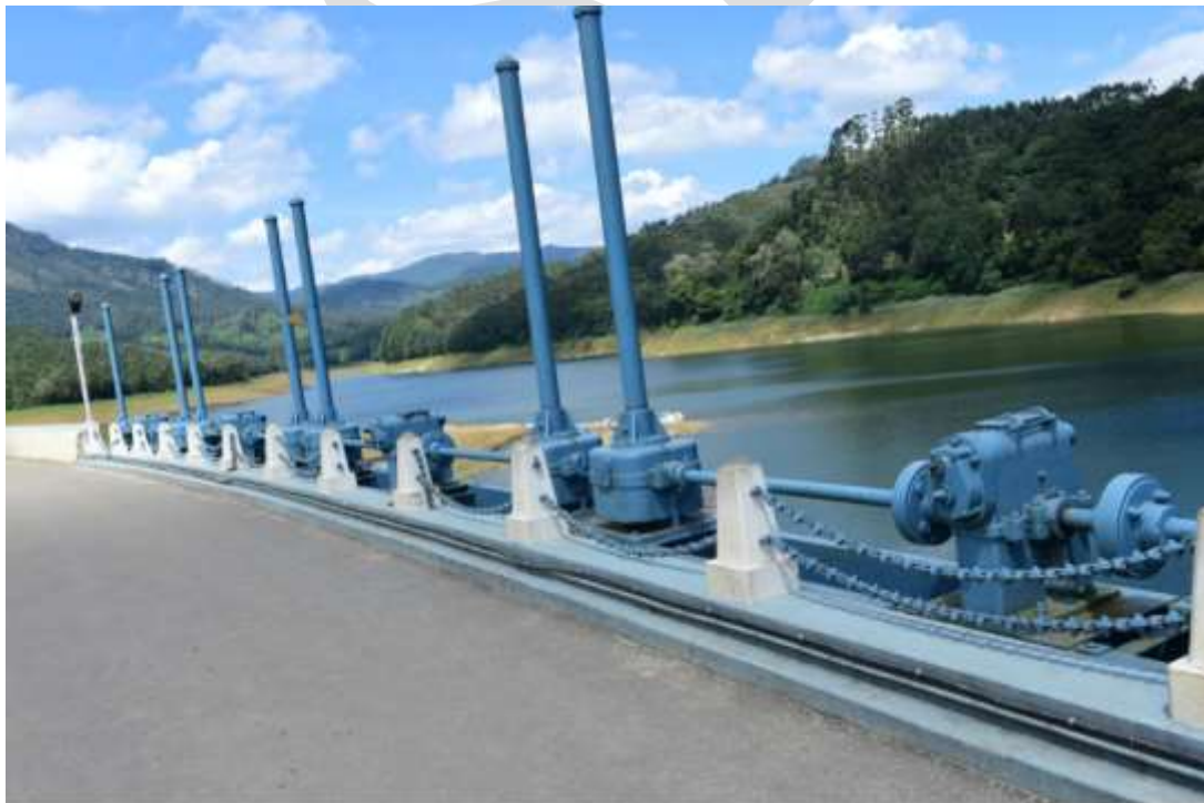
Fig 2.7 Screw hoists for vertical lift spillway gates
