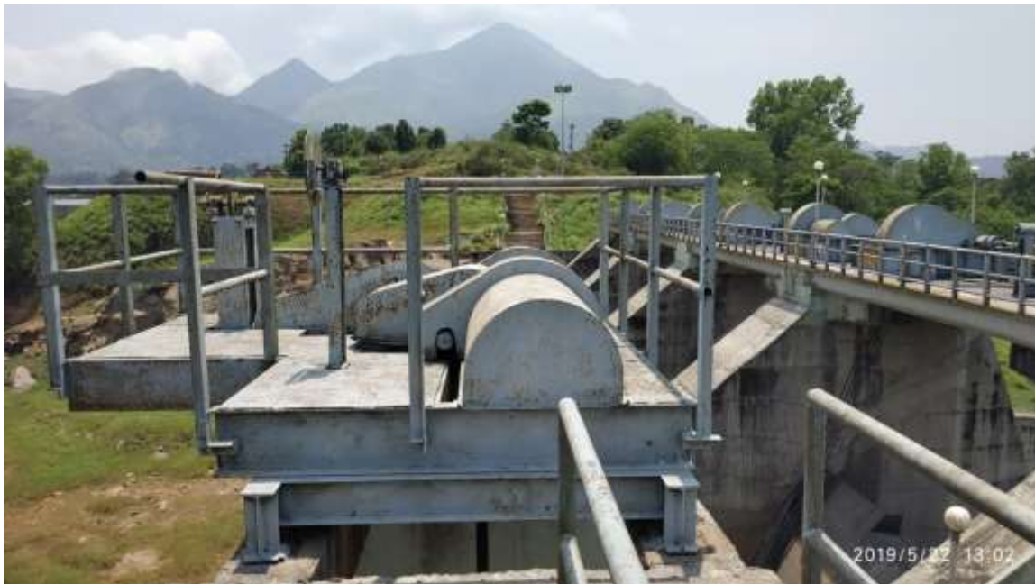
Fig. 2.8 River Outlet Vertical Gate Hoisting Mechanism
