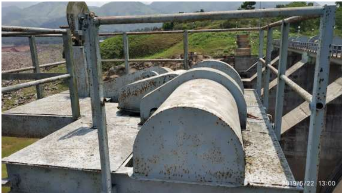
Fig. 2.9 Irrigation Outlet Vertical Gate Hoisting Mechanism
