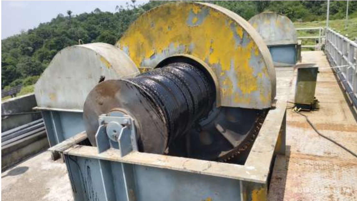
Fig 2.5 Radial Gate Hoist Rope Drum
