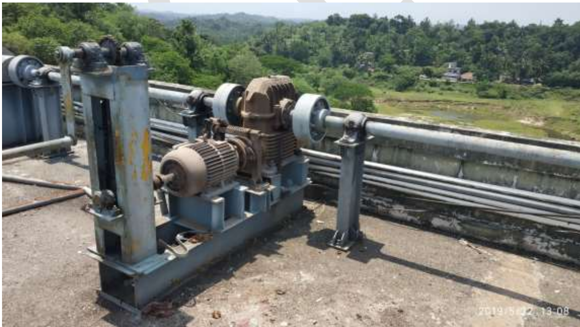
Fig. 2.4 Radial Gate Hoisting Mechanism
