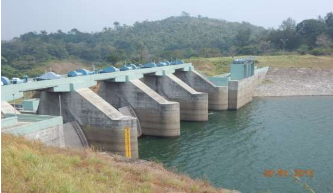
Fig 2.3 Radial Gates Hoist Bridge
