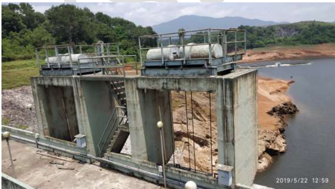
Fig. 2.10 Hoisting Mechanism of Vertical Gates of River and Irrigation Outlets
