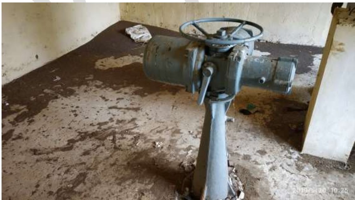
Fig. 2.7 River Outlet Disperser Valve Opening Mechanism
