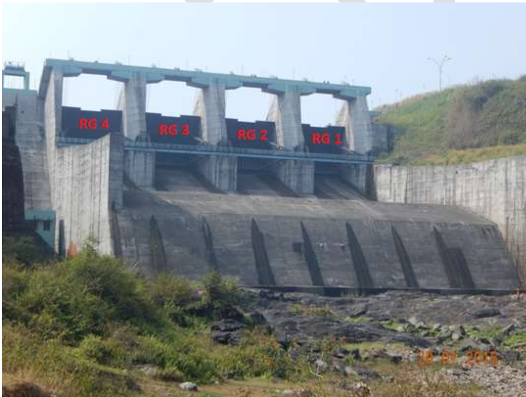
Fig 2.25 Spillway Radial Gates
