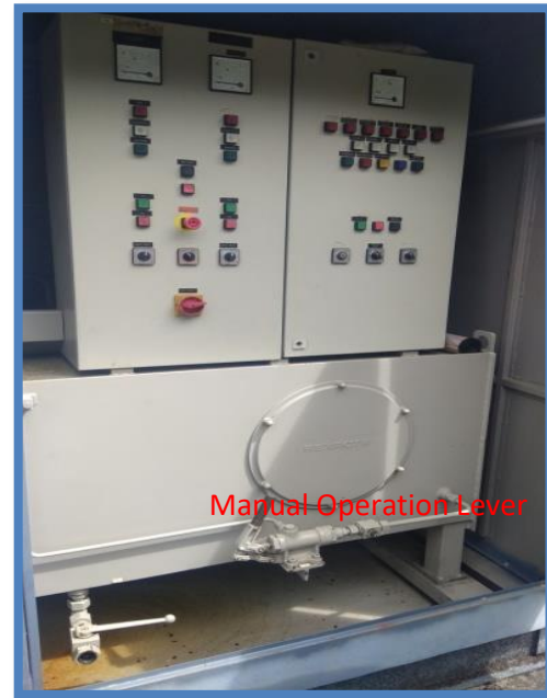
Fig 2.12 Photograph of Control panel Lower vent
