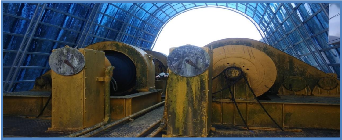
Fig 2.17 Photograph of Intake Hoisting Arrangements
