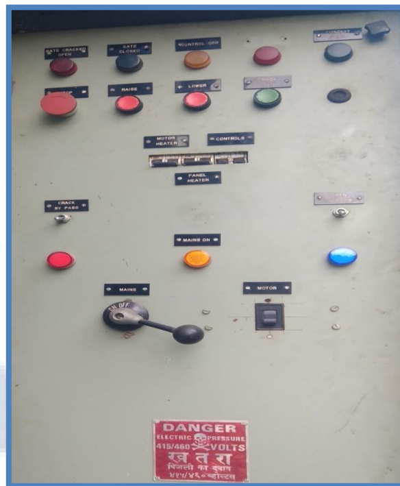
Fig 2.18 Photograph of Intake Hoisting Arrangements of Control Panel
