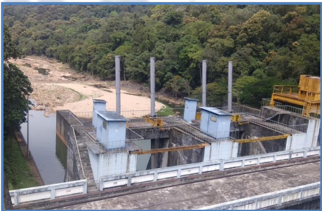
Fig 2.10 Photograph Showing Hoisting arrangements of Radial Gate for Lower Vent
