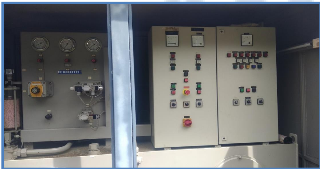
Fig 2.13 Photograph of Control panel of Lower vent(a)
