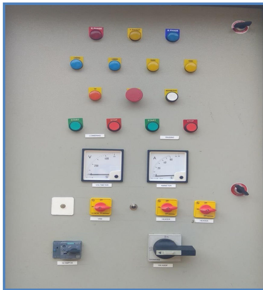
Fig 2.8 Photograph Showing Control Panel of Radial gate for Upper vent
