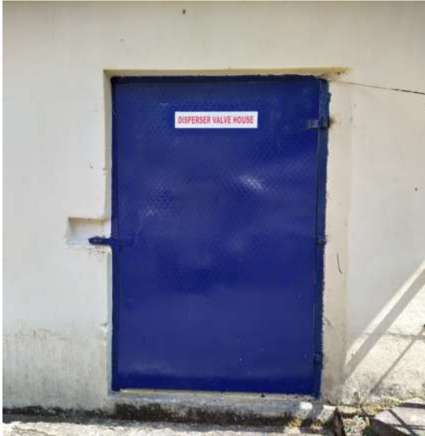
Fig 2.8 Dispenser valve house
