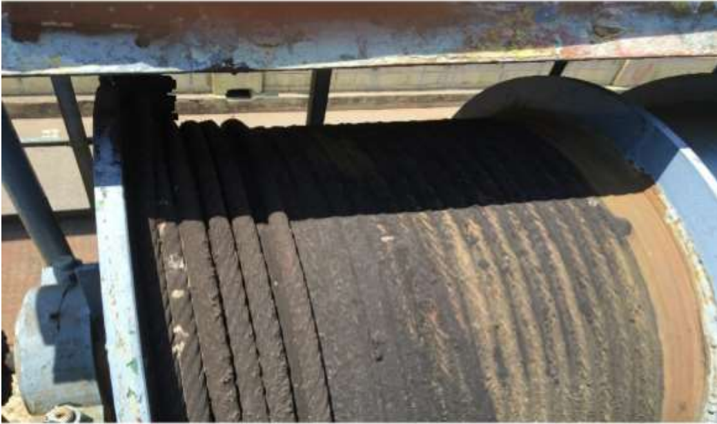
Fig 2.23 Intake rope drum hoist
