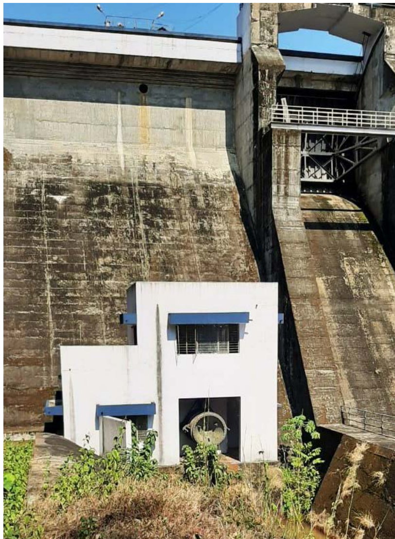
Fig 2.4 Disperser valve downstream
