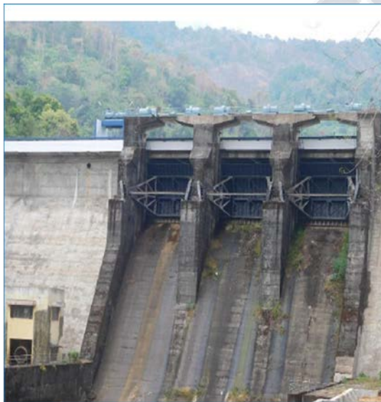
Before - No roofing to the hoist of radial gates
