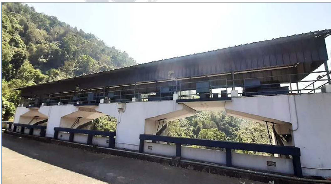
Fig 2.10 Moozhiyar Dam Spillway Hoist Mechanism
