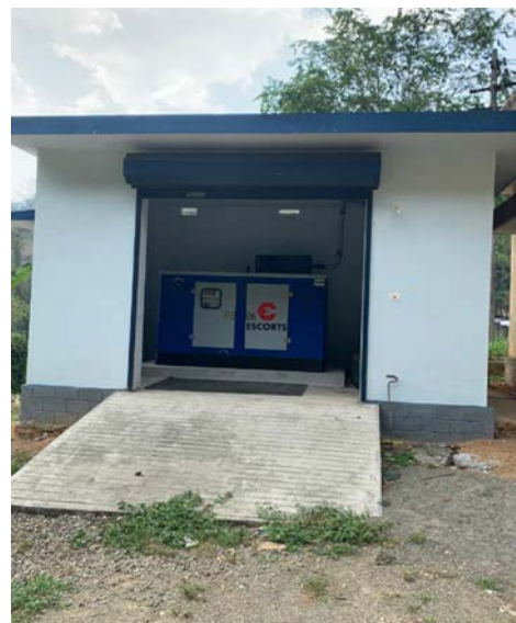
After - Construction generator room
