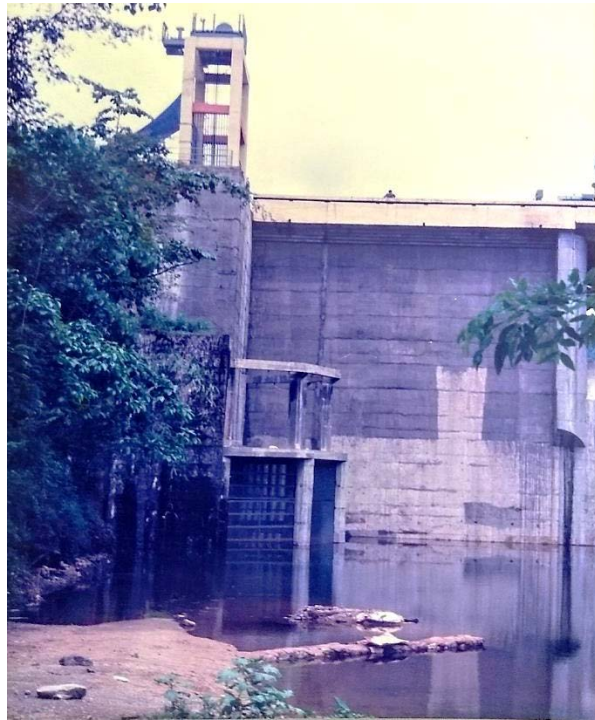
Fig 2.15b Power Intake and Trash rack
