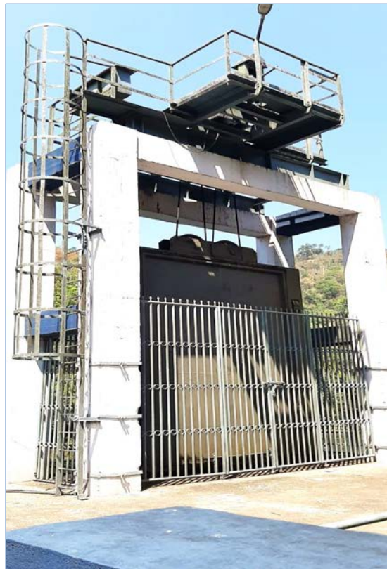
Fig 2.13a Intake gate and hoist
