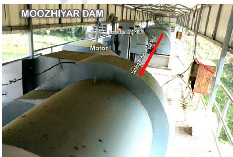
Fig 2.11c Radial Gate hoist mechanism
