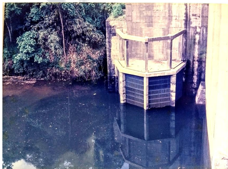
Fig 2.16 Moozhiyar Dam Trash rack at intake
