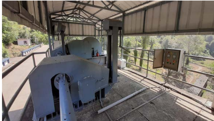
Fig 2.11a Radial Gate hoist mechanism
