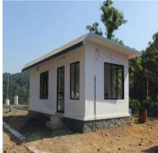
Monitoring cabin – Final stage
