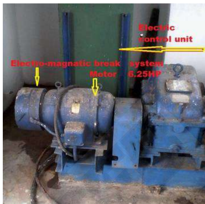
Fig 2.3 IC Tunnel Hoist Motor
