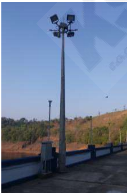
High mast light
