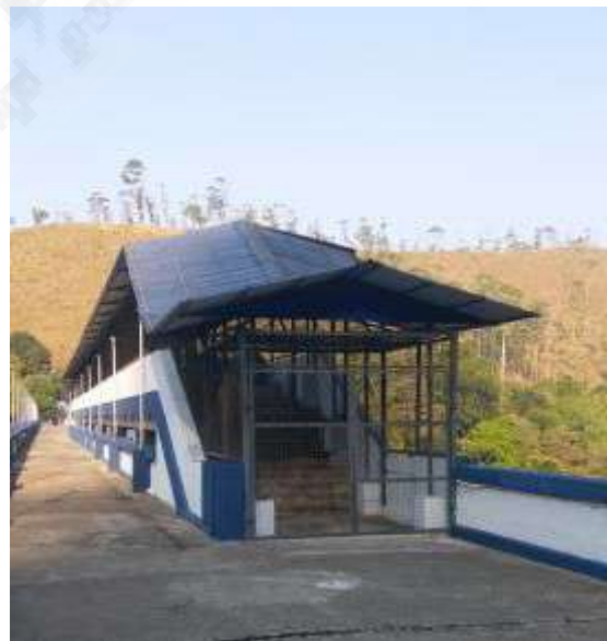
After – Supply and Erection of Roofing to hoist of Pamba Dam radial gate
