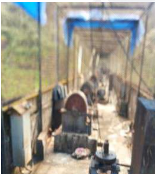
Before – Supply and Erection of Roofing to hoist of Pamba Dam radial gate
