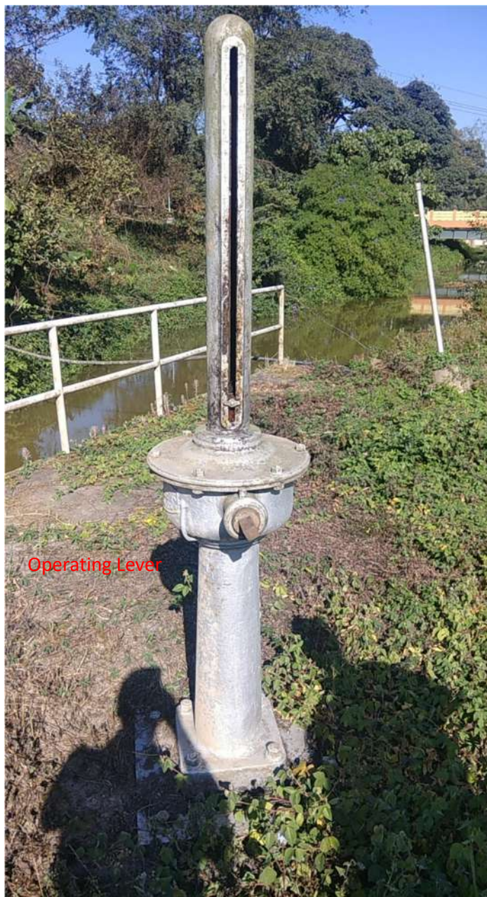
Fig 2.7 Sluice Gate Operating arrangements
