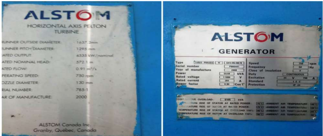
Fig 1.15 Name plate of Turbine and Generator (Unit I, II& III)
