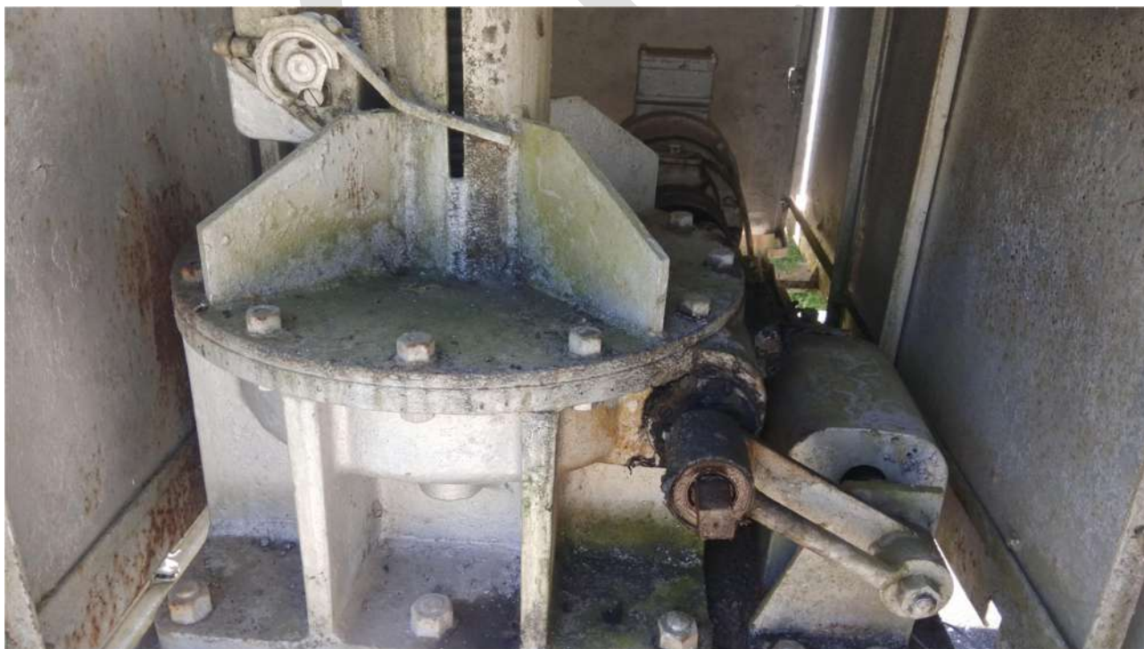
Fig 2.14 Tunnel Inlet – Hand Operating Arrangements
