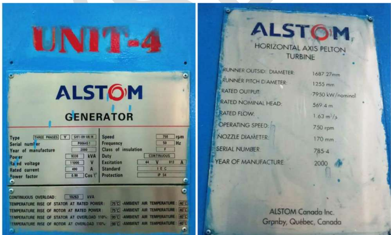
Fig 1.14 Name plate of Turbine and Generator (Unit IV, V & VI)
