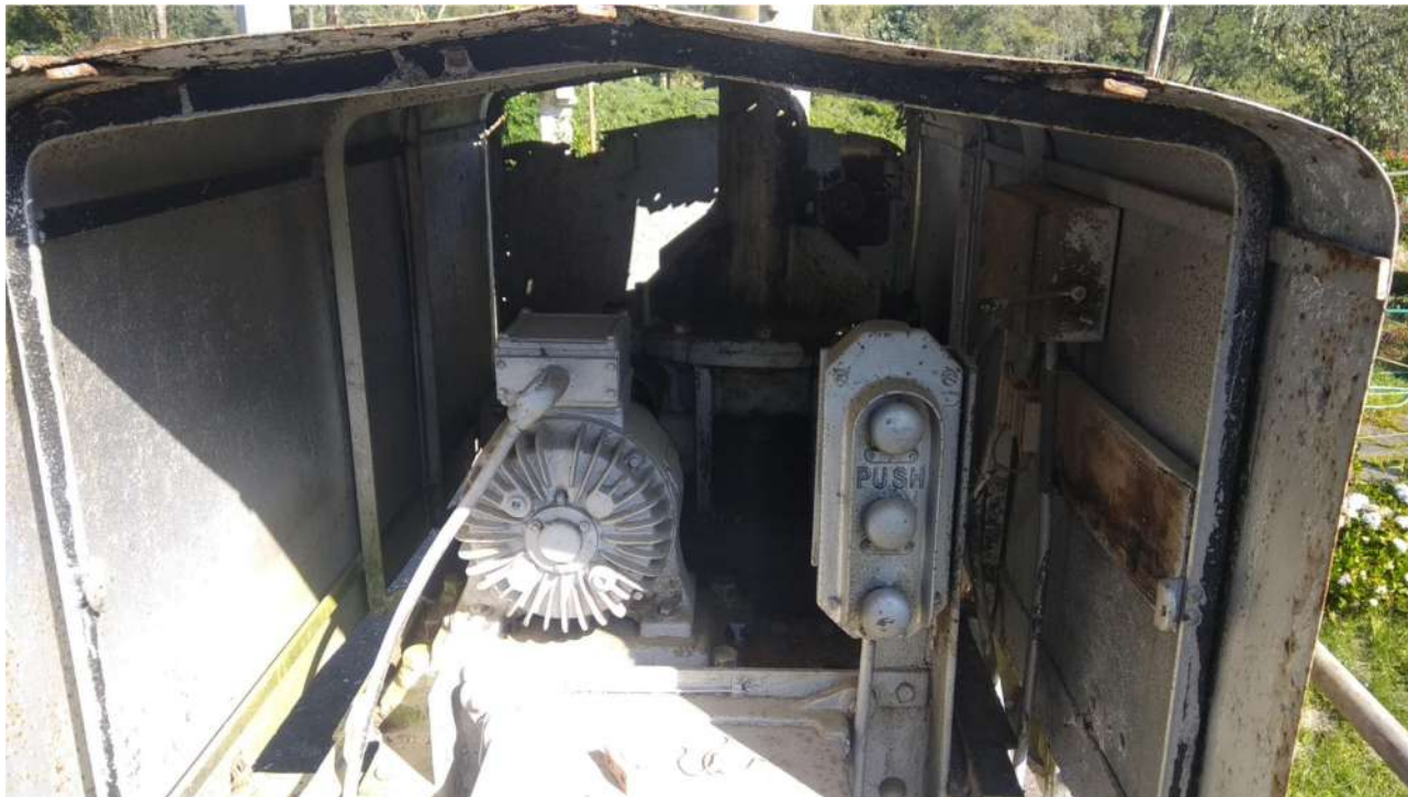
Fig 2.13 Tunnel Inlet – Operating Switches
