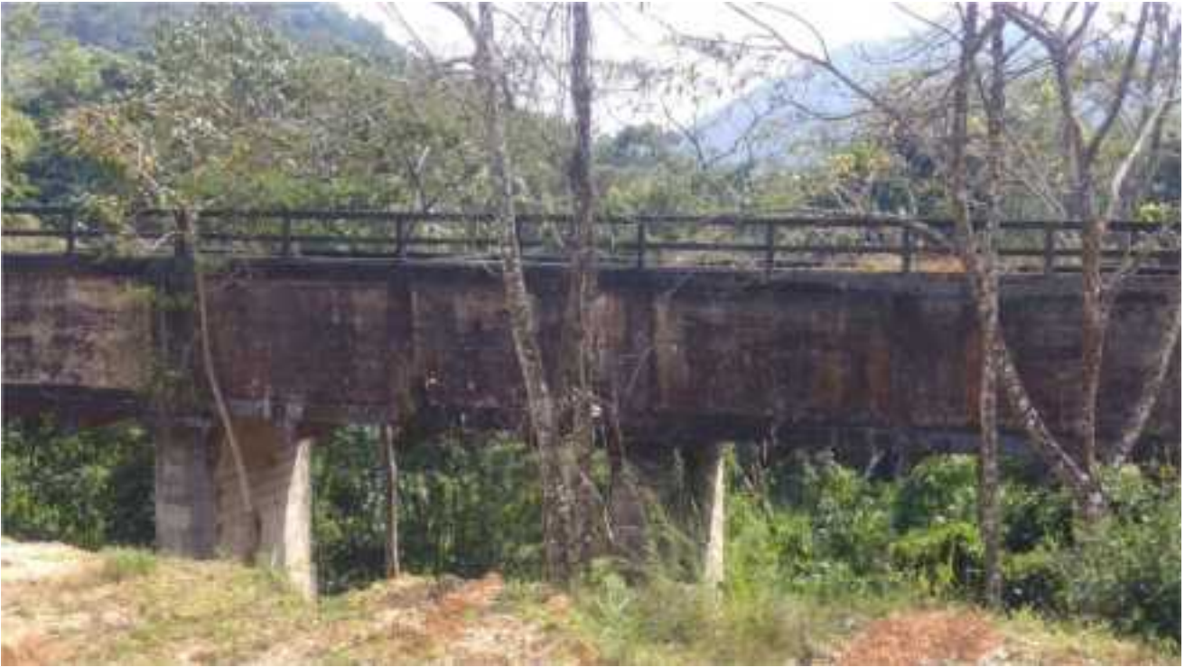
Fig 1.10 – RCC Aqueduct as a part of Power Channel No.1 to convey water to pump house
