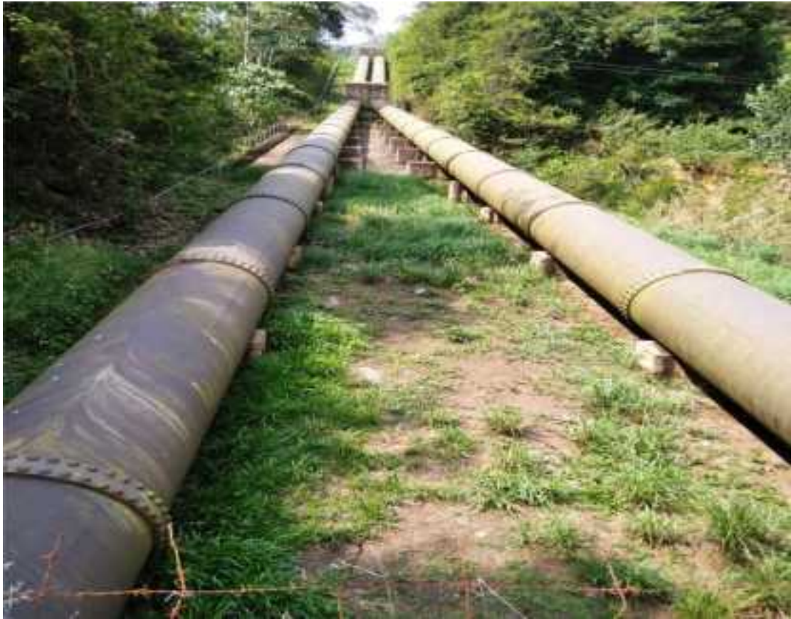
Fig 1.21 – High Pressure Pipe (Penstock)
