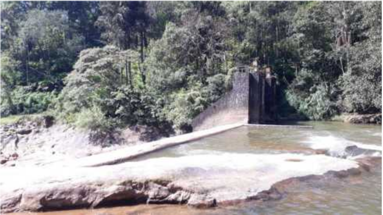
Fig 1.8 – Pickup Weir near to Pallivasal PH to collect spillover from RA Head Works
