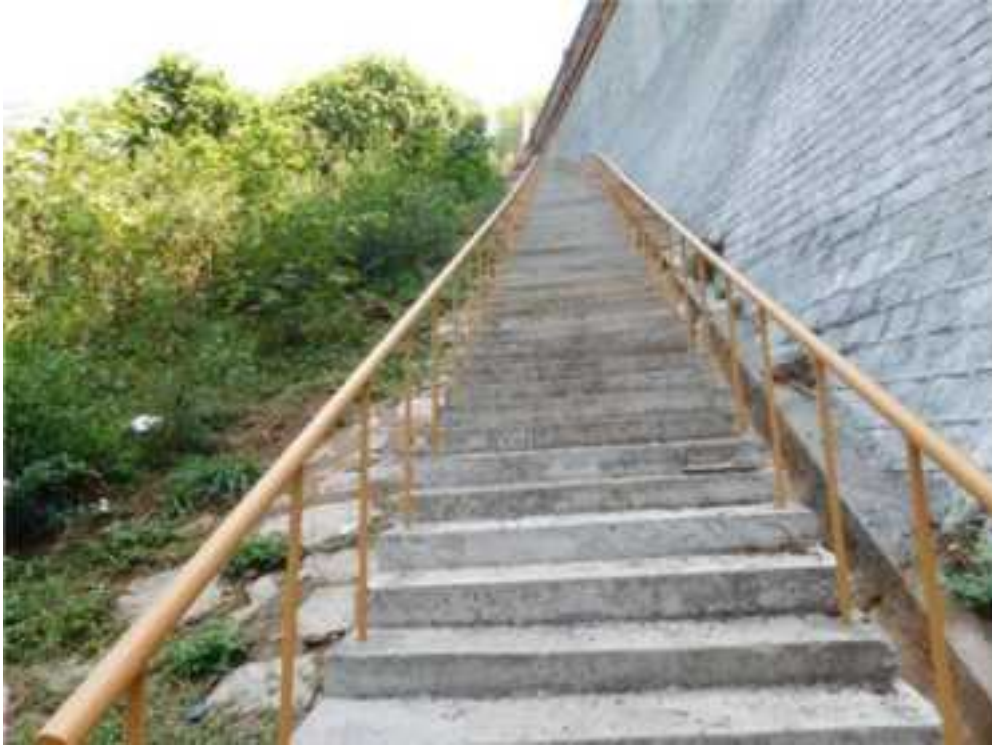
Fig 6.13 Newly constructed Steps to Dam gallery from right bank of Dam top
