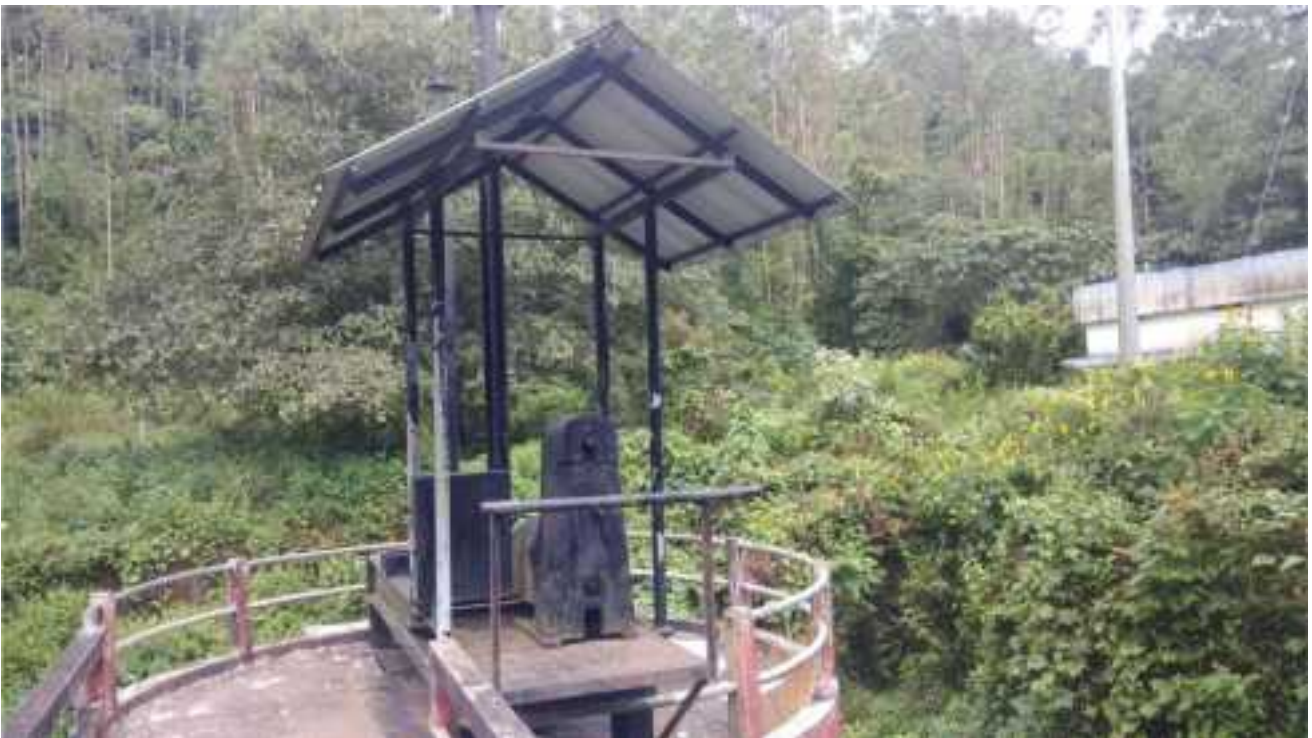
Fig 1.15 – Close up view of Intake Hoisting arrangements
