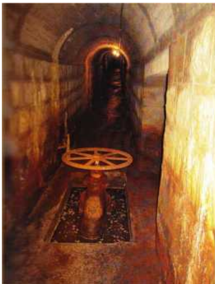
Fig 2.3 Hand operated wheel valve for scour vent in the inspection gallery
