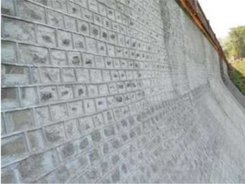
Fig 6.12 Raised and cut pointing for Dam body at downstream face of Dam
