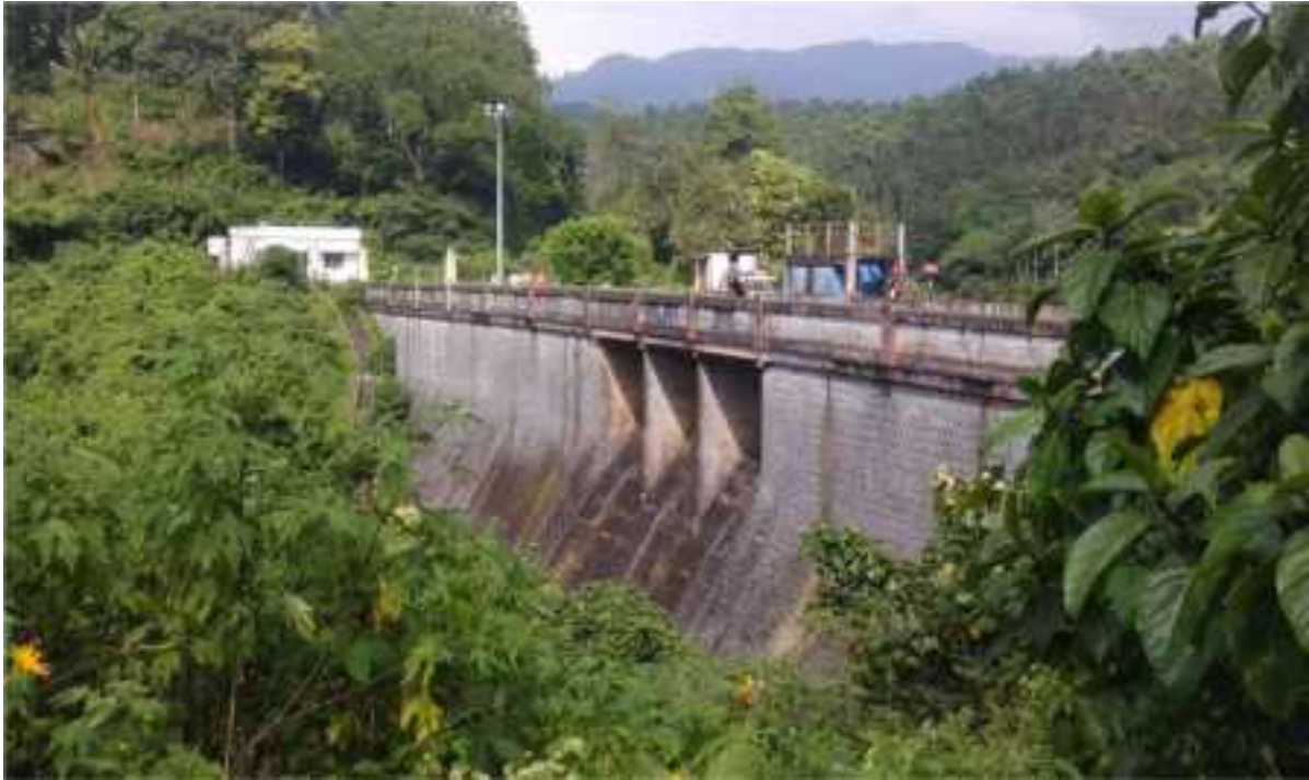
Fig 6.8 Photograph showing High mast light at Dam top and Painting of dam body
