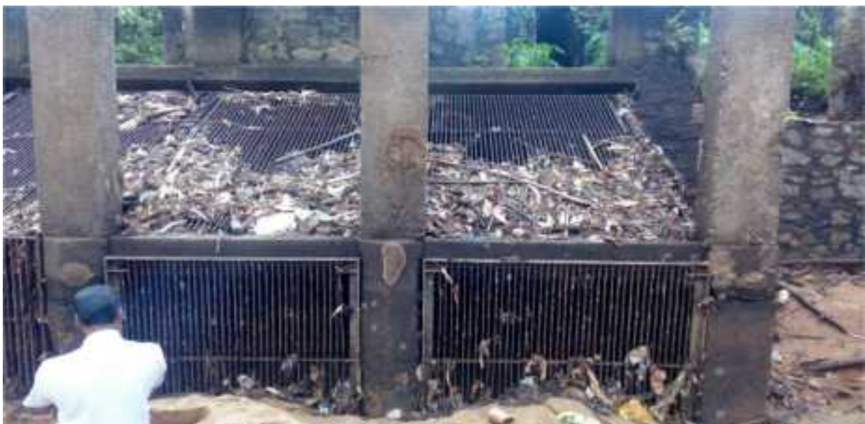
Fig 2.7 Intake trash rack
