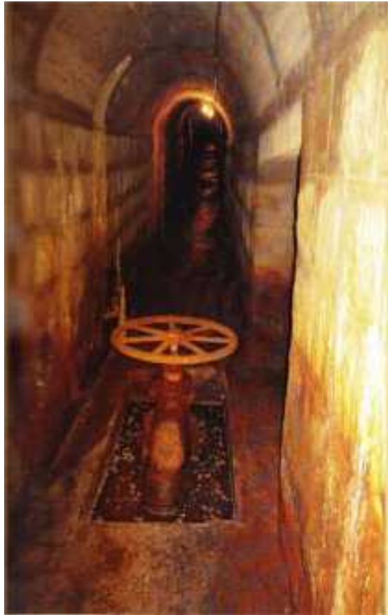
Fig 6.3 Photograph showing Sluice Wheel Valve
