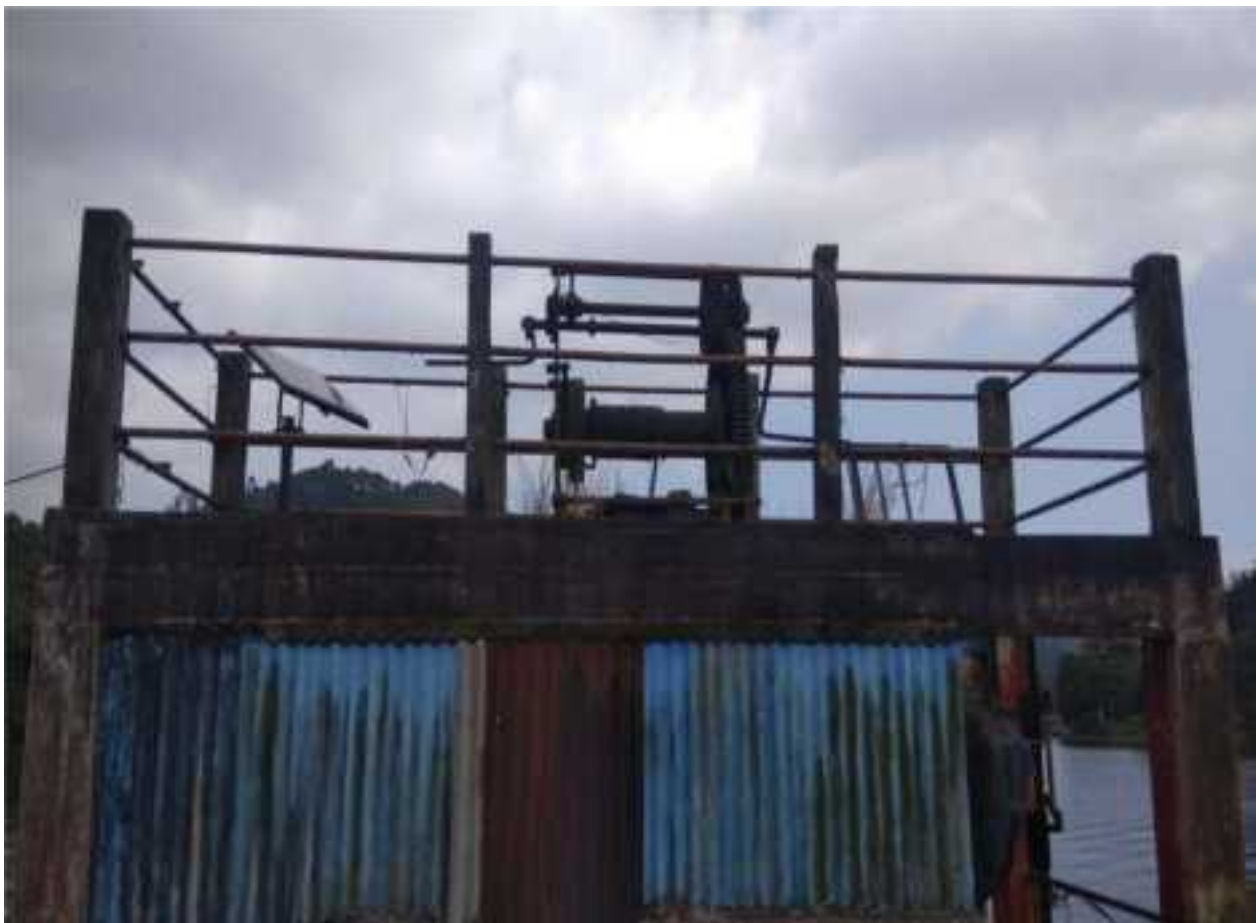
Fig 2.2 Hoisting winch of emergency gate
