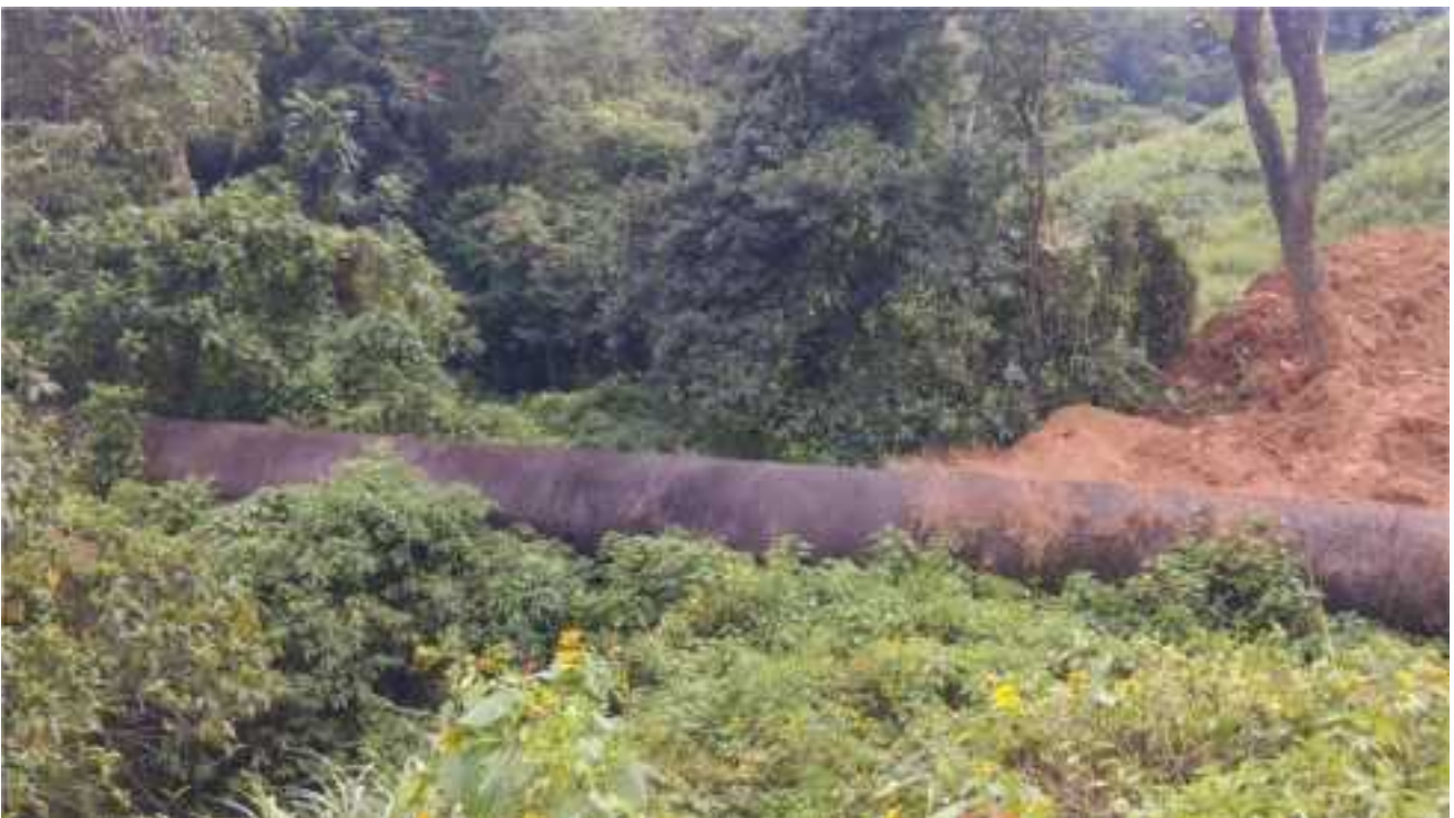
Fig 1.12 – Pumping line from Pump House to Tunnel 1
