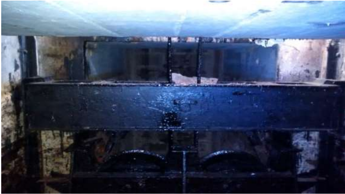
Fig 6.3 Emergency gate guides before replacement
