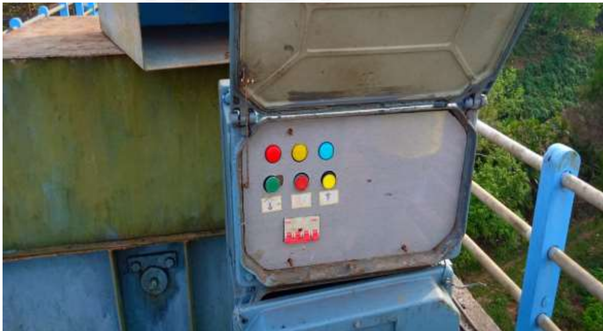
Fig 2.7 Control panel of Hoisting mechanism
