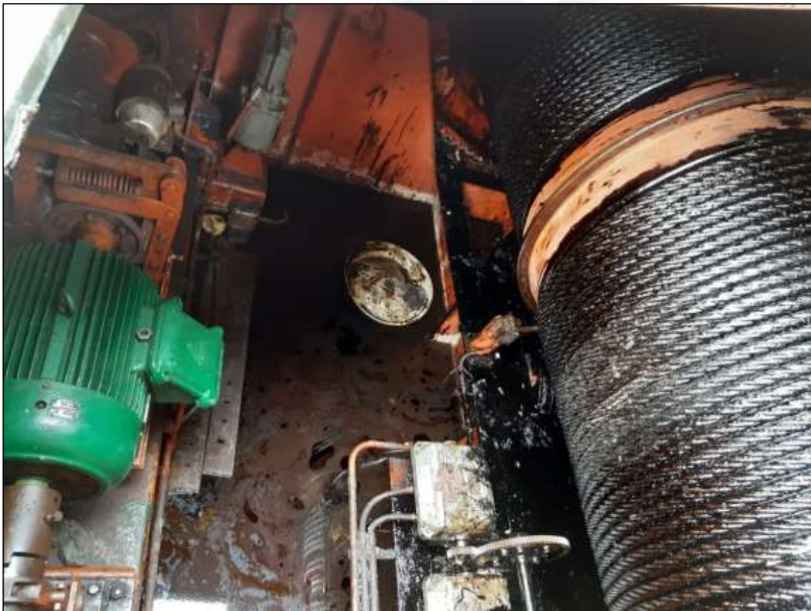
Fig 2.26 Wire rope and motor in intake gate hoist chamber
