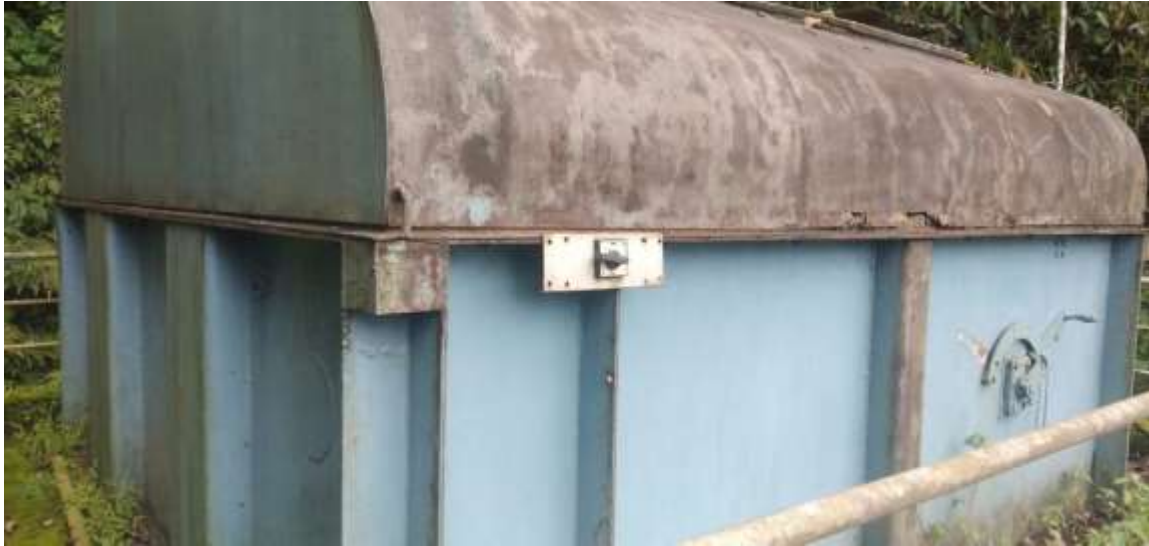
Fig 2.25 Intake gate hoisting structure
