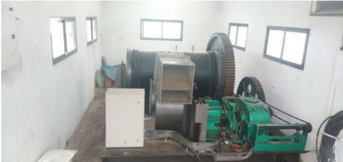
Fig 1 Emergency gate hoisting mechanism
