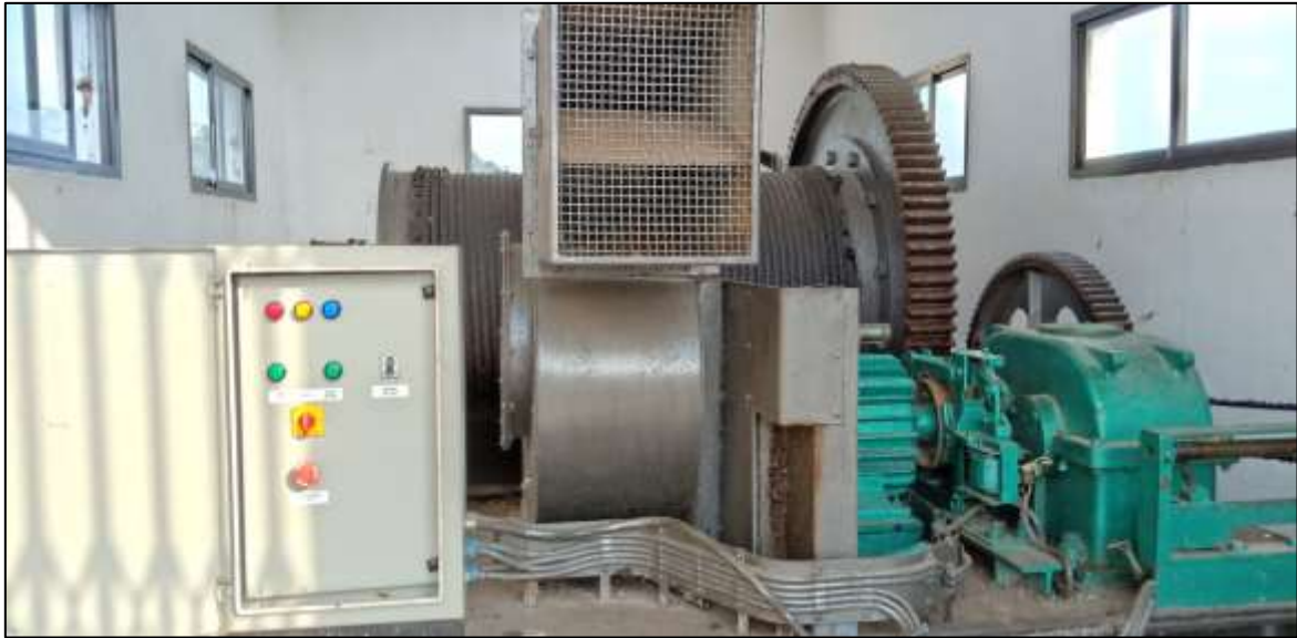
Fig 2.15 Rope drum of Emergency gate
