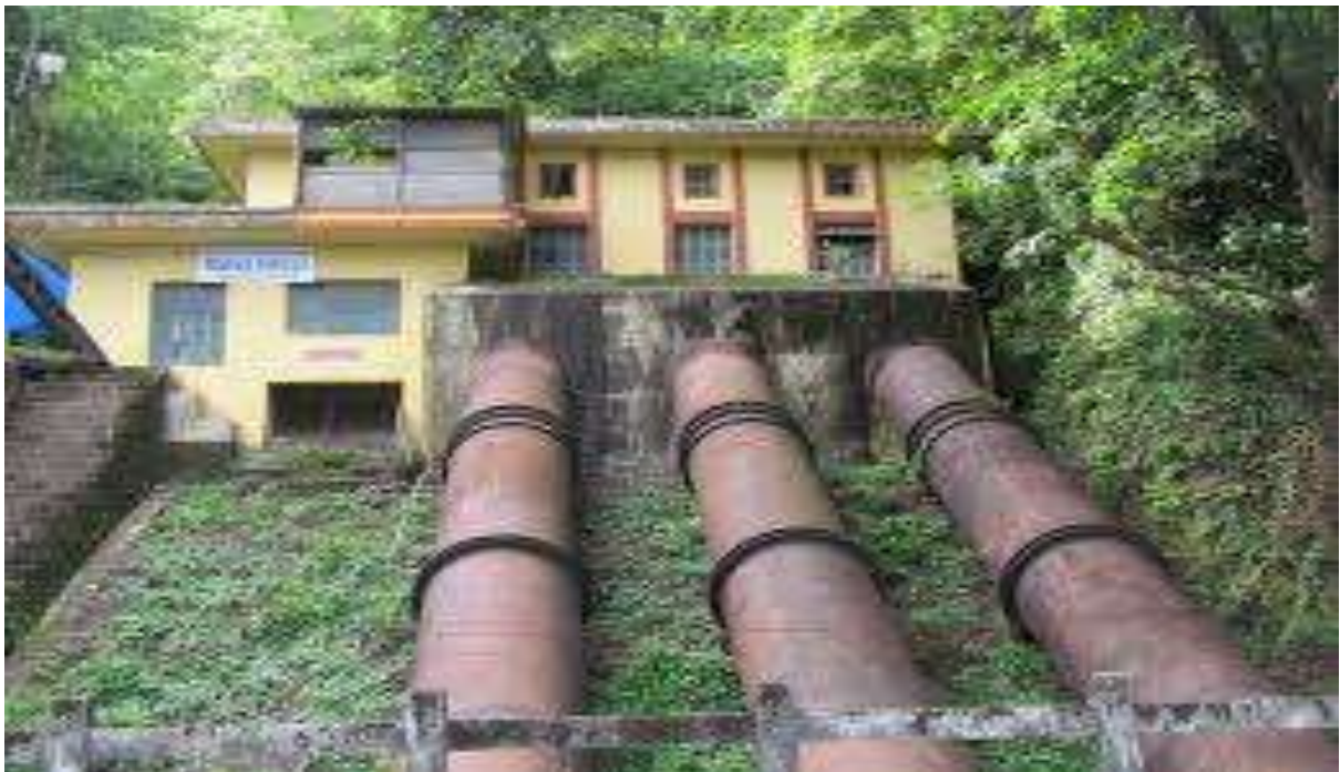
Fig 2.28 Penstock and valve house
