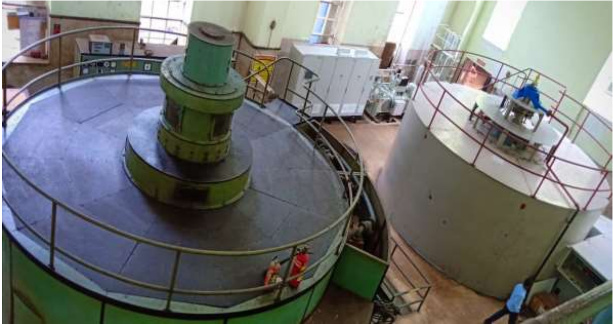
Fig 2.30 Power House Turbine
