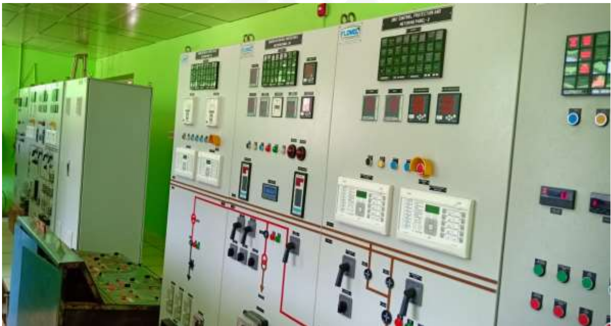
Fig 2.31 Power House Control panels
