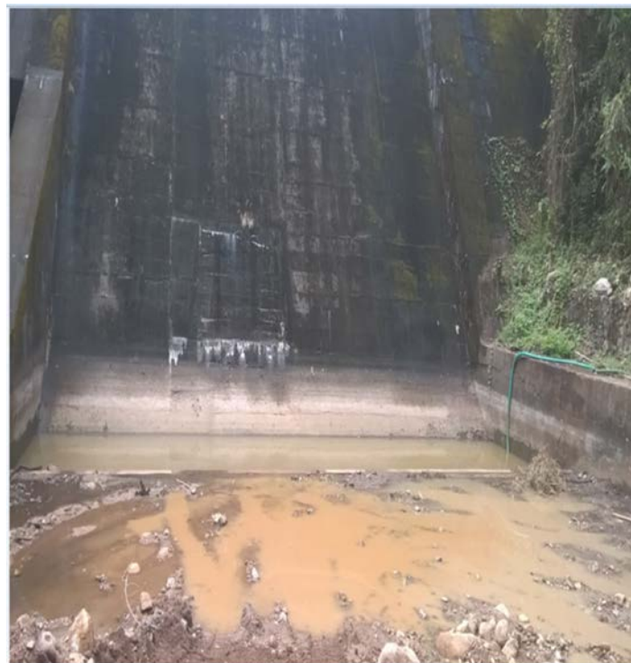
After - Removal of debris/ loose stones from downstream of spillway channel of Veluthode dam
