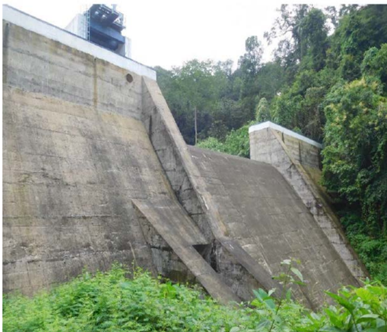
After - Pressure washing the downstream face and allied structures of Veluthode dam
