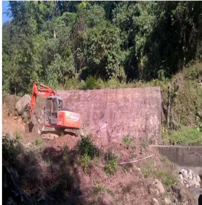
Before - Removal of debris/ loose stones from downstream of spillway channel of Veluthode dam
