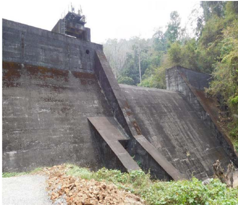
Before - Pressure washing the downstream face and allied structures of Veluthode dam
