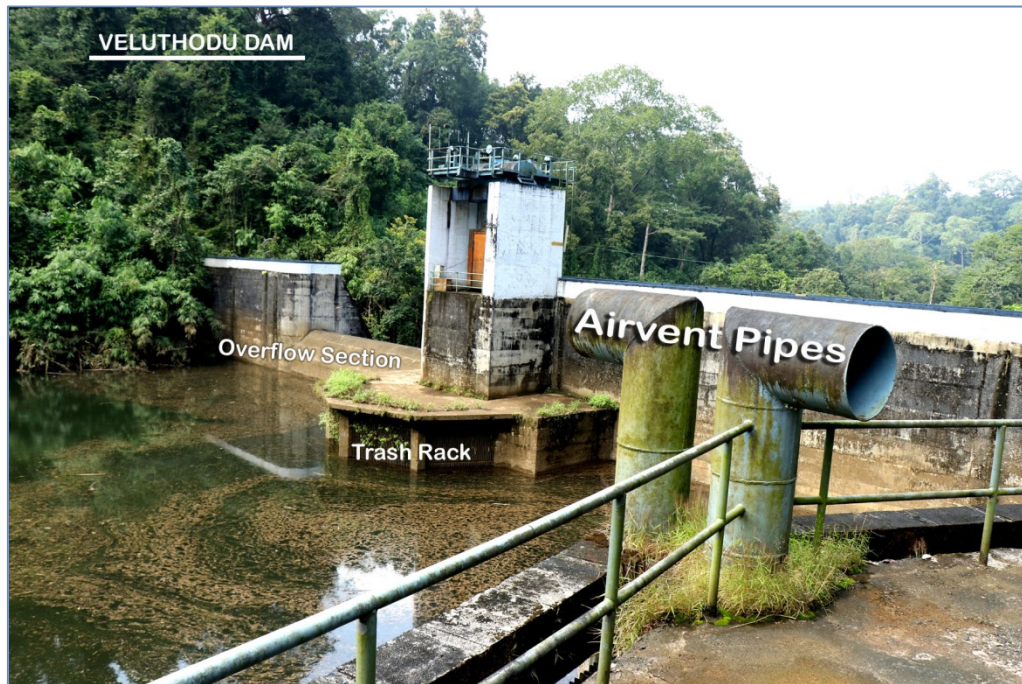
Fig 2.8a River sluice/ emergency gate hoist structure
