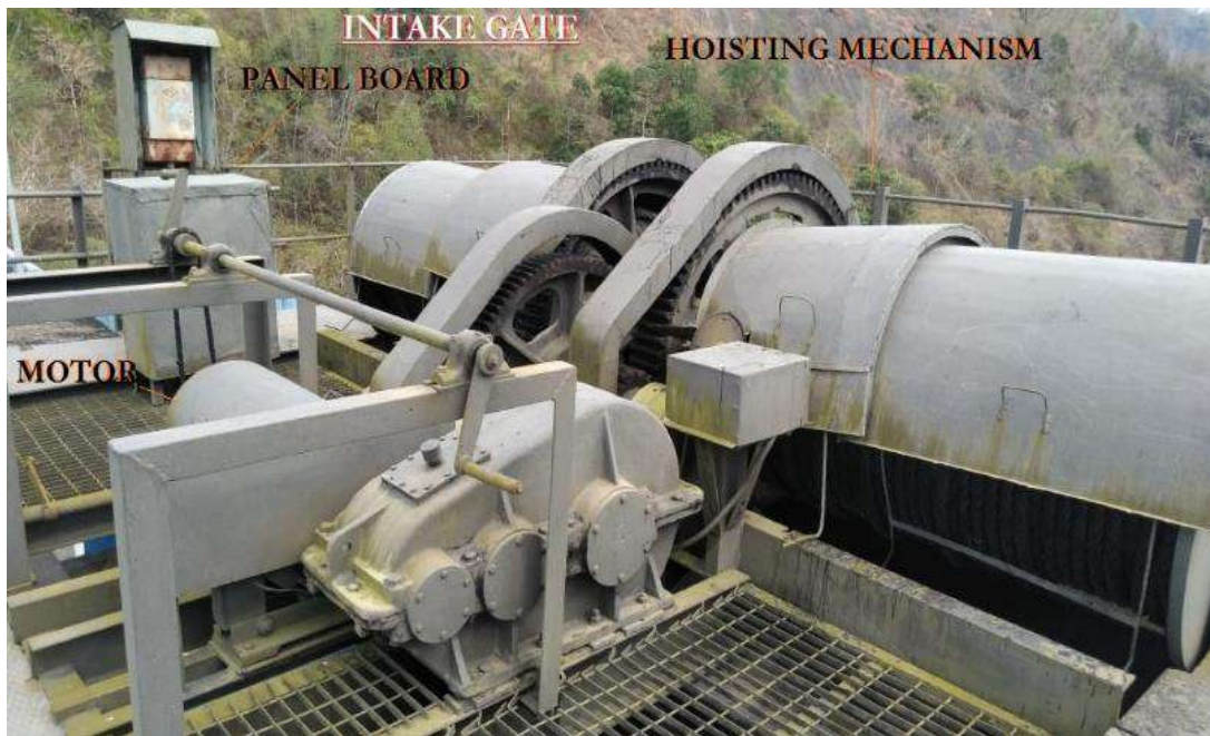
Fig 2.11 Idamalayar Dam Intake Gate Hoist Mechanism
