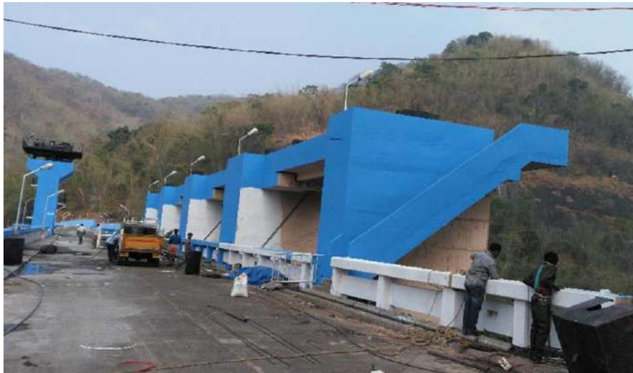
Fig 2.3 Radial Gates Hoist Bridge
