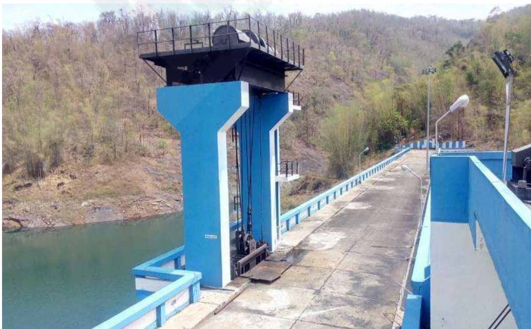
Fig 2.10 Idamalayar Dam Vertical Gate
