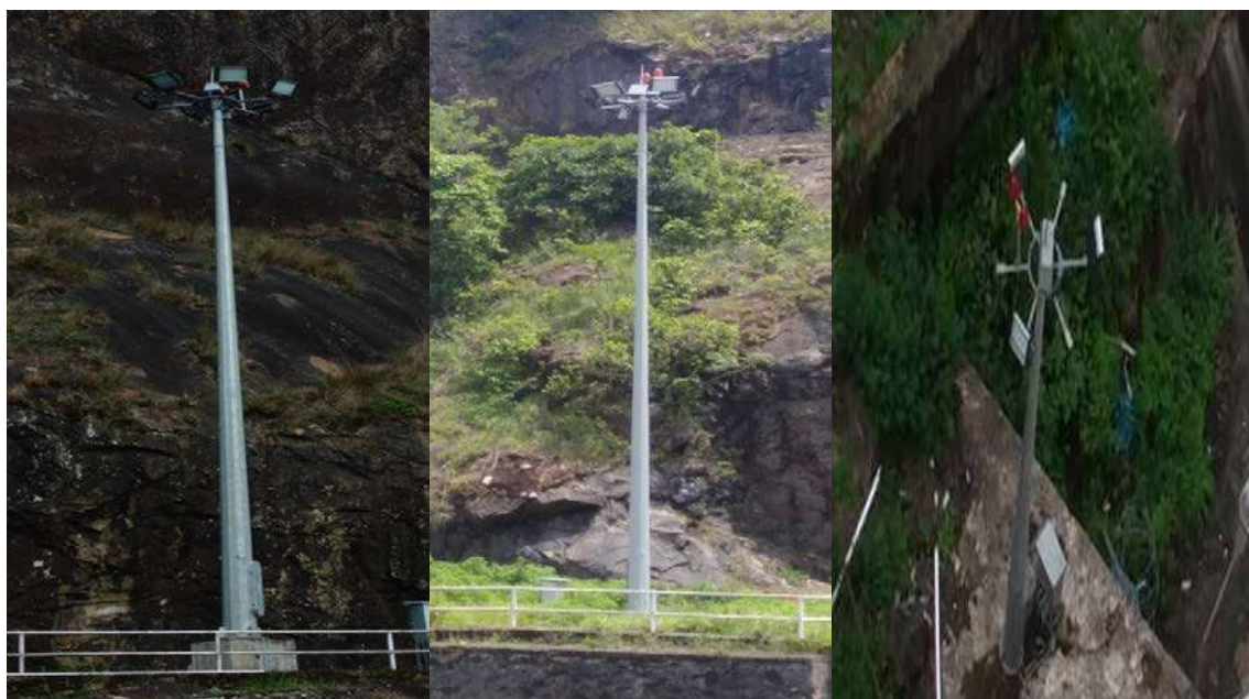
High mast lights in Idukki dam premises
