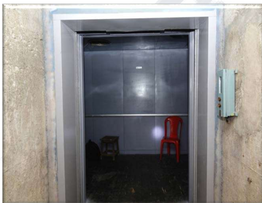
Fig 1.26 Elevator at Cheruthoni dam
