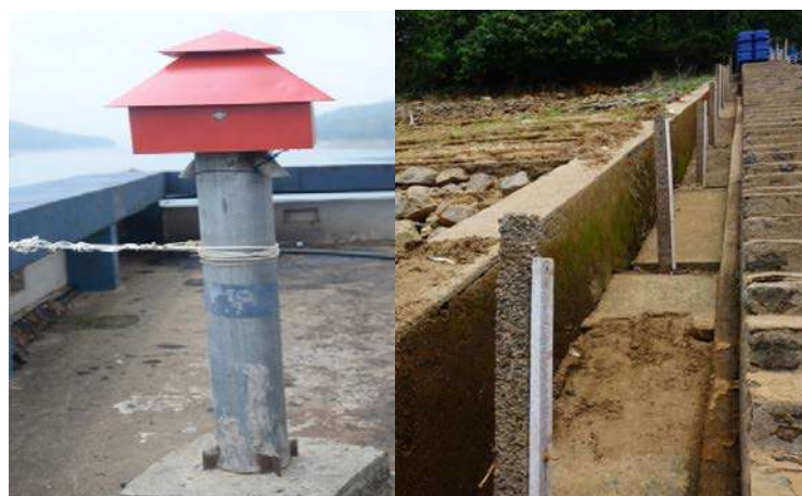
Fig 5.9 Automatic water level reader and manual reading scales
