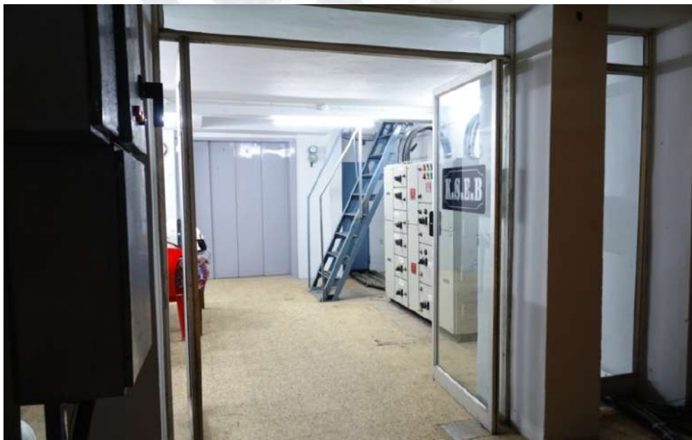
Fig 1.18b View of lift entrance and electrical panel board
