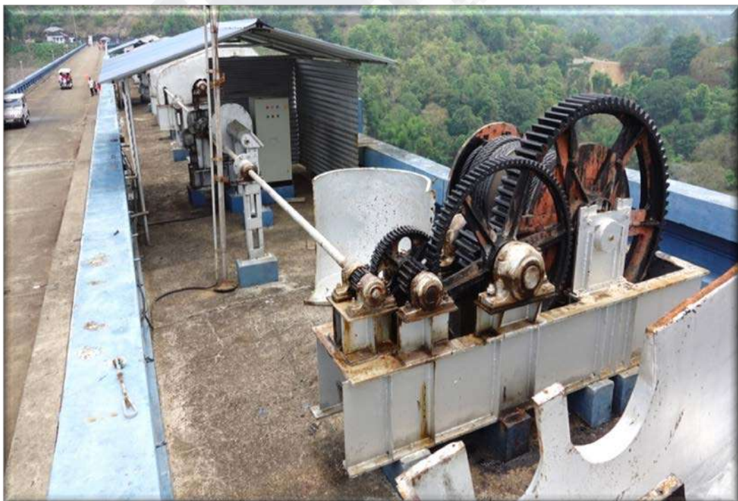
Fig 2.10 View of Gate operation Gear mechanism and Electric control panel
