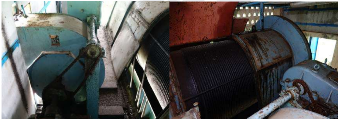
Fig 2.21c Intake Gate Hoist
