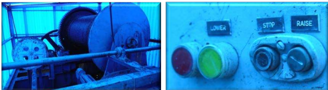
Fig 2.16 Hoist drum, gear system and panel board for sluice gate operation
