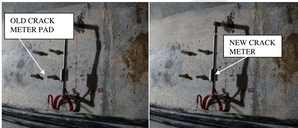
Crack meter old and new fixed at old cracked wall of gallery at El.2300 ft
