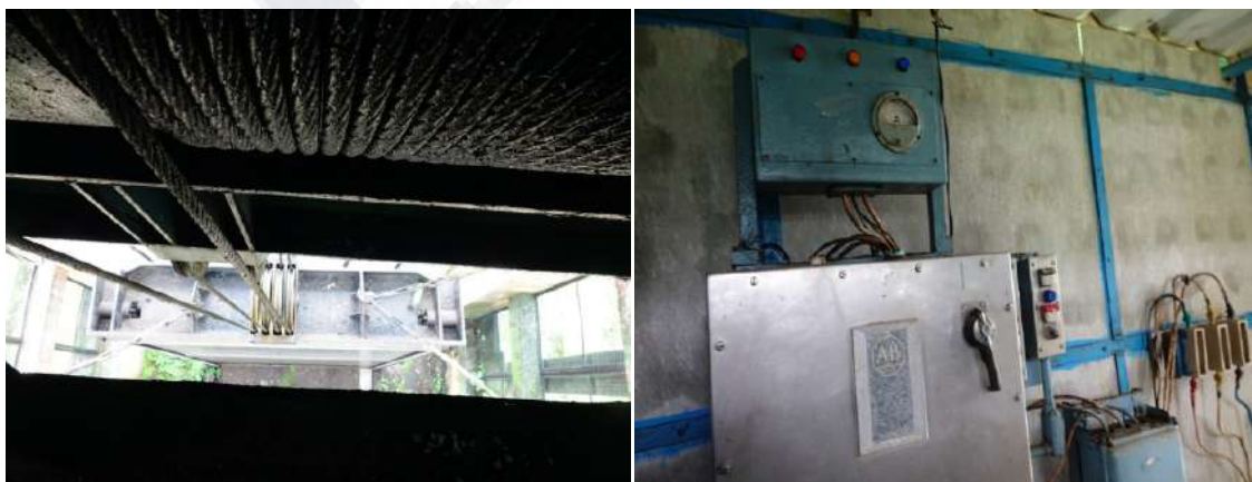
Fig 2.22 Intake Gate Hoist Wire rope and Operating Control
