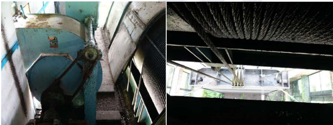
Control shaft Intake Gate hoist
