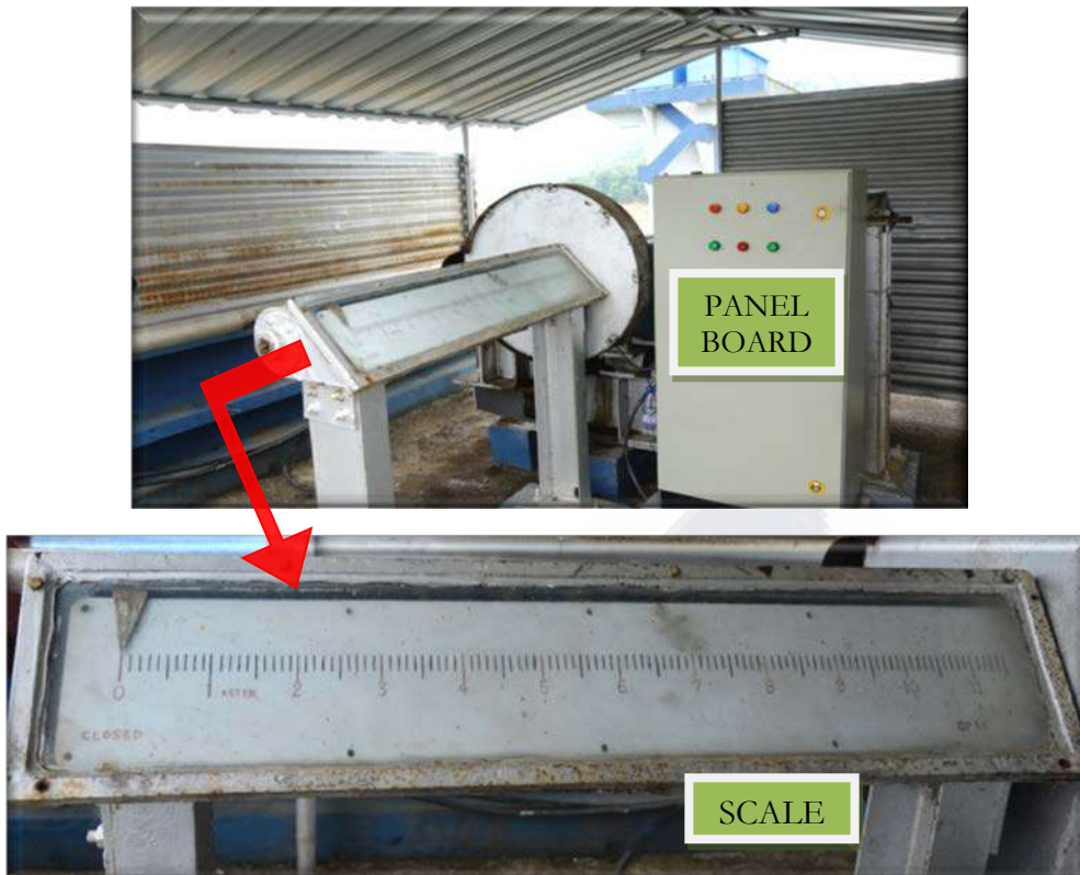
Fig 2.11 Control panel and measuring scale for the radial gates hoist
