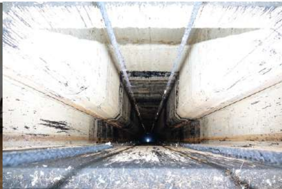
Emergency gate wire rope
