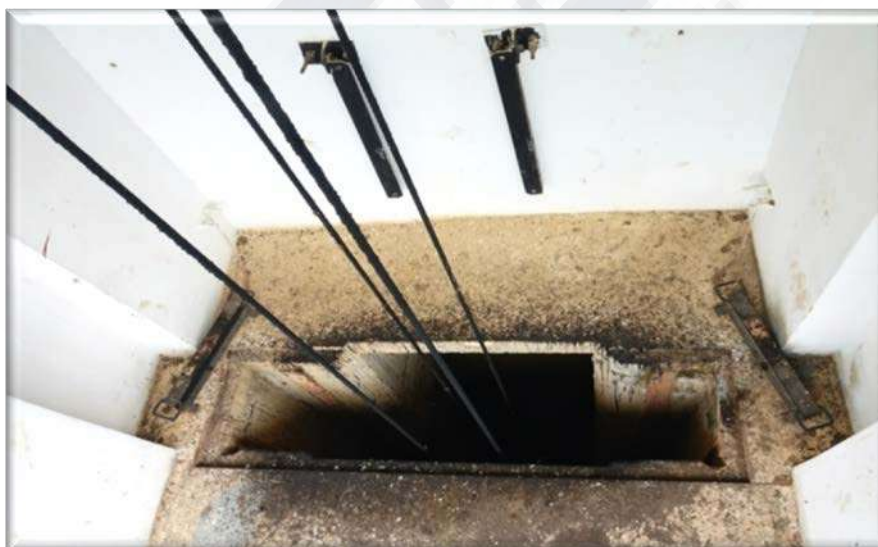
Fig 1.33 Emergency gate hoist
