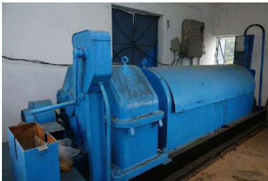
Emergency Gate Hoisting Machine
