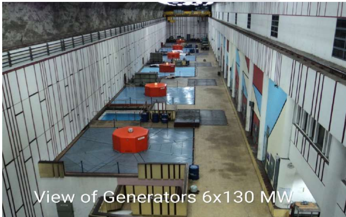
Fig 1.36 IHEP Power House Generators
